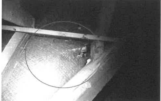
Torn/ worn roofing felt indicative of roost site
