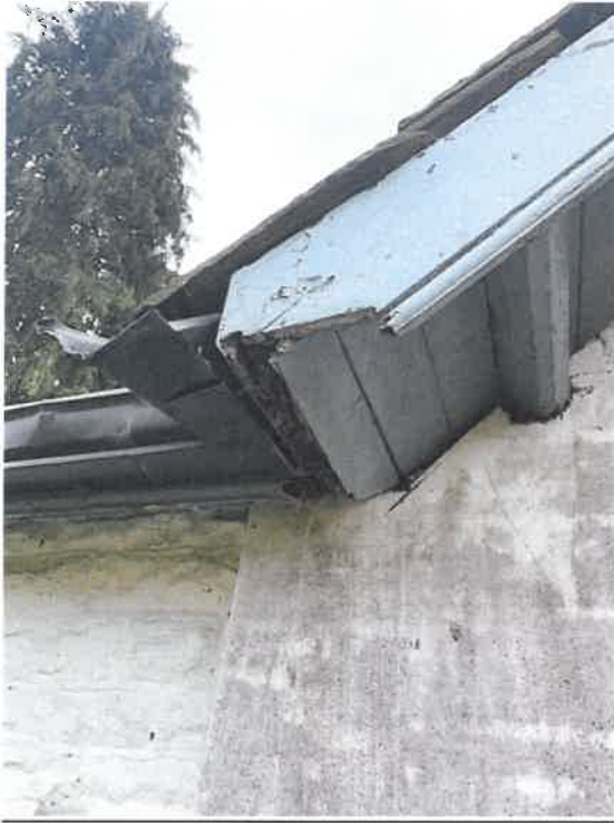
Image 1 shows defective soffits and fascia and the damaged rainwater drain
