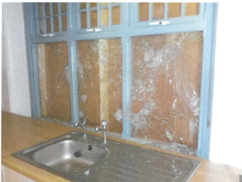
Image 6 shows the existing glazing smashed and boarded up, its proposed to be replaced by bullet proof glass.
