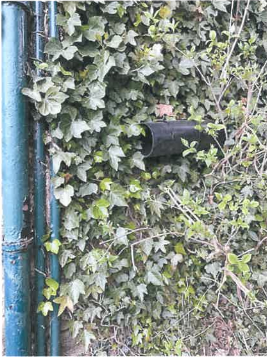
Image 3 and 4 show the damaged existing uPVC soil stack
