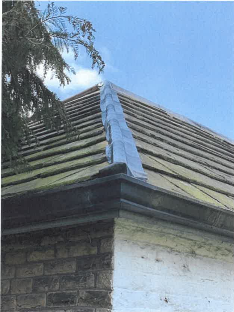
Image 5 shows the existing temporary flashing over the wood core rolls on the hips and ridge. It is proposed to replace this with zinc flashing.
