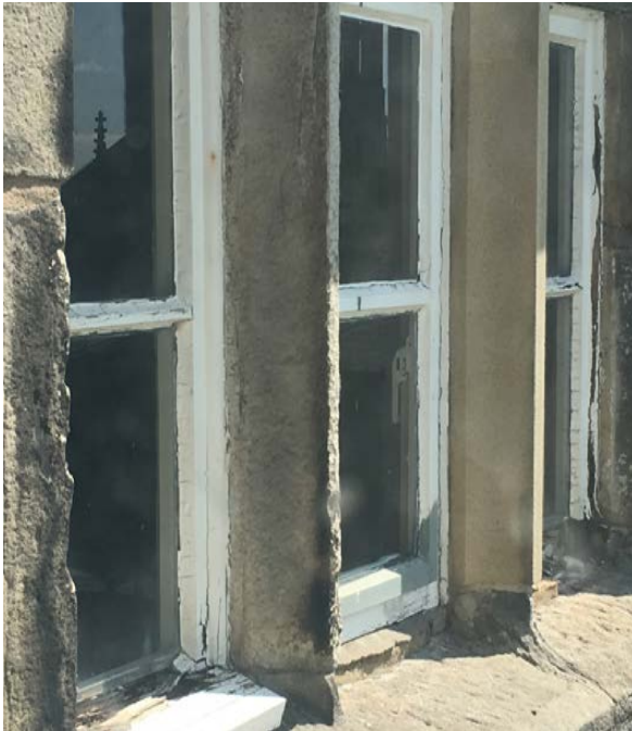
Above: badly weathered modern timber window
