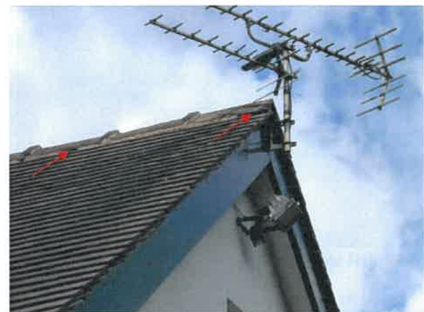
Location of mortar gaps under ridge tiles, requiring supervised removal of features under precautionary measures.
