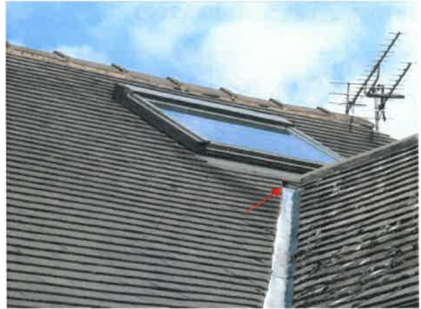
Location of small hole beneath Velux window on southern elevation and mortar gaps under ridge tiles, requiring supervised removal of features under precautionary measures.
