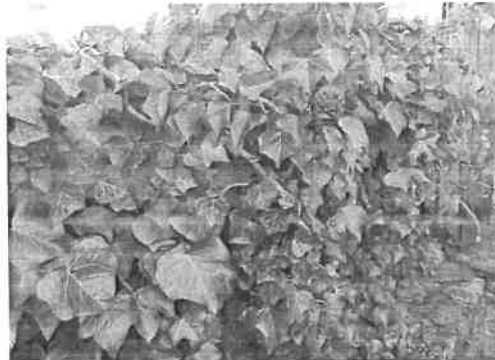
Photo 12: Dense ivy cladding on the western boundary of roof terrace.
