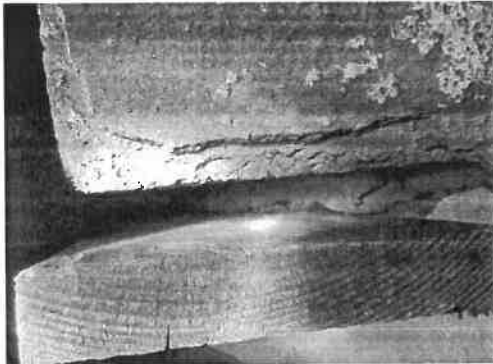
Photo 9: 'V' shaped gap between the soffit and soffit box
