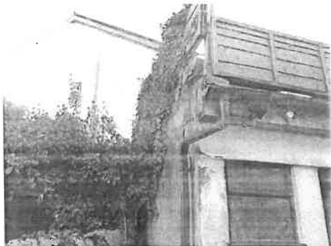
Photo 11: Overhanging ivy cladding on the western side of the building which densely covers the neighbouring shed. The outbuilding wall narrows against the neighbouring wall.
