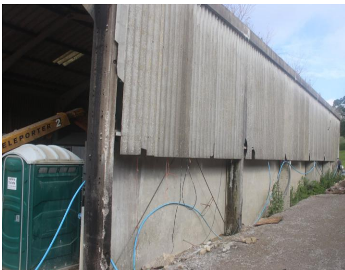
Barn 1 with corrugated fibre cement sheet walls and cast concrete base walls, concrete portal frame.
