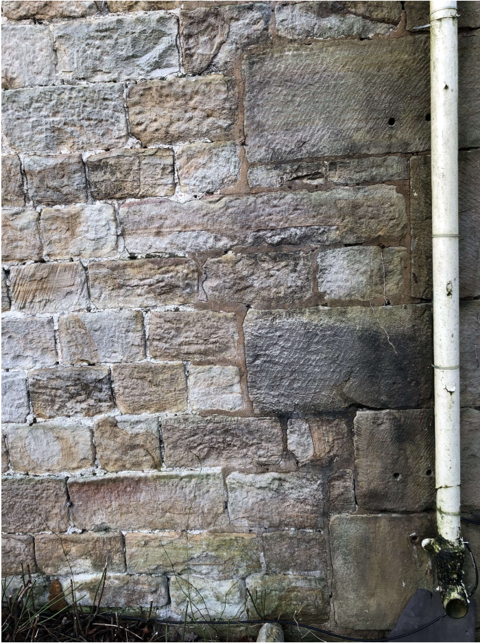
Photo c) Cement mortar causing damage to the softer sandstone
