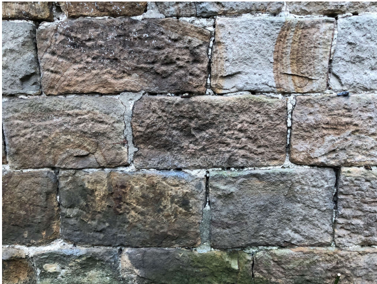
Photo b) Worn lime mortar which requires maintenance
