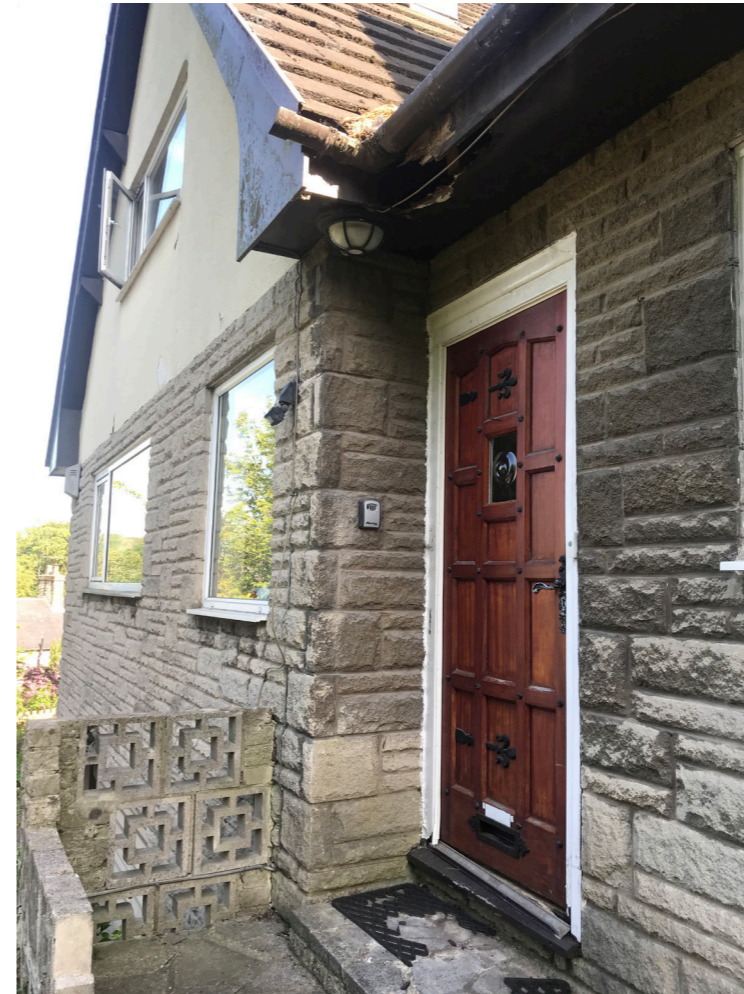
Existing principal elevation showing rotten soffits
