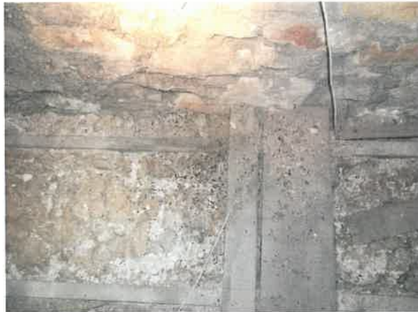
Plate 3. Bat droppings at eastern gable end (zone 1)
