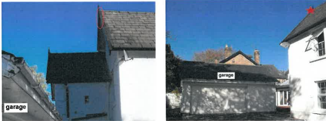
Close proximity of roost (illustrated in red) to garage as seen from south-west and south-east
