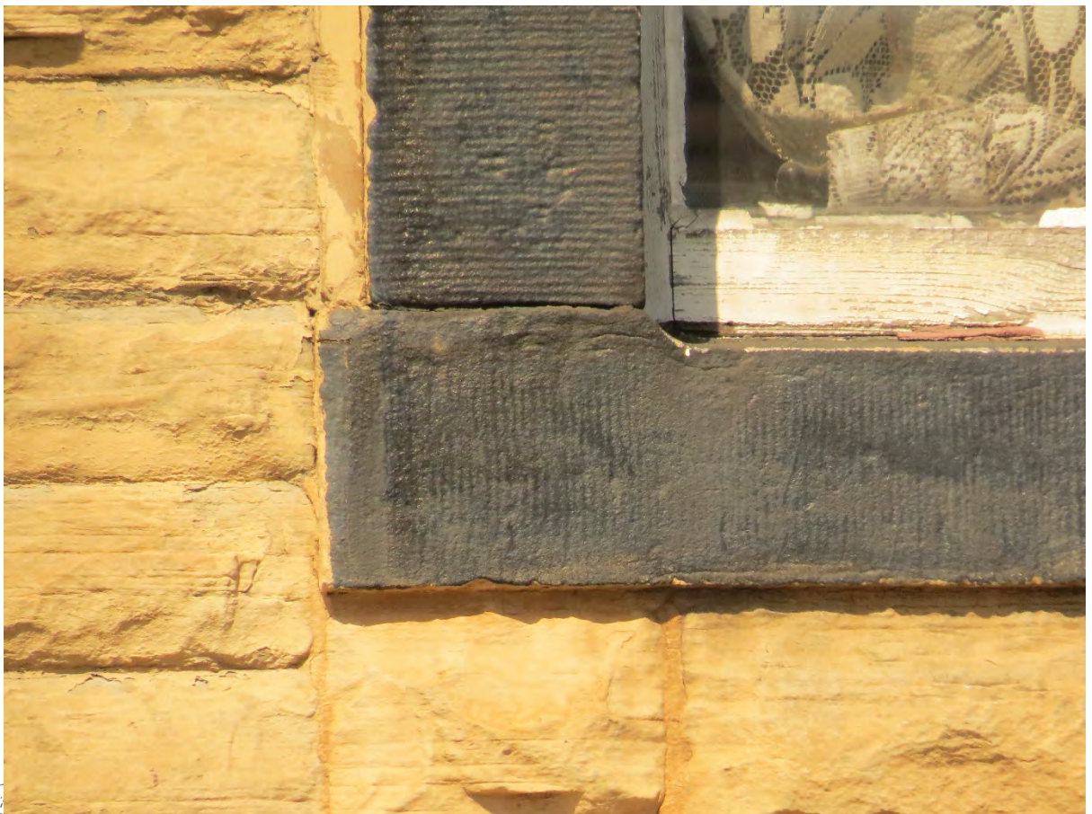
8 – Stone lintels and window settings have no suitable gaps.
