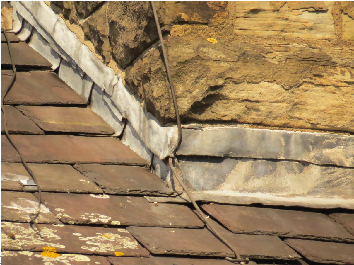
6 – Leadwork is tight with no suitable gaps.
