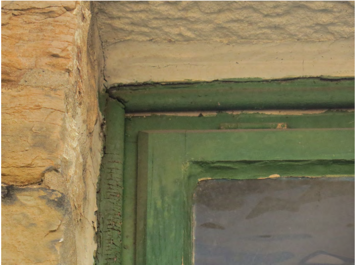
7 – Window and door frames are tightly sealed into stonework with no suitable gaps.
