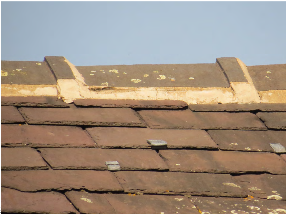
4 – Ridge tiles are tightly cemented in place with no suitable gaps.
