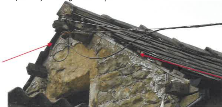
Gaps at abutment with slates
