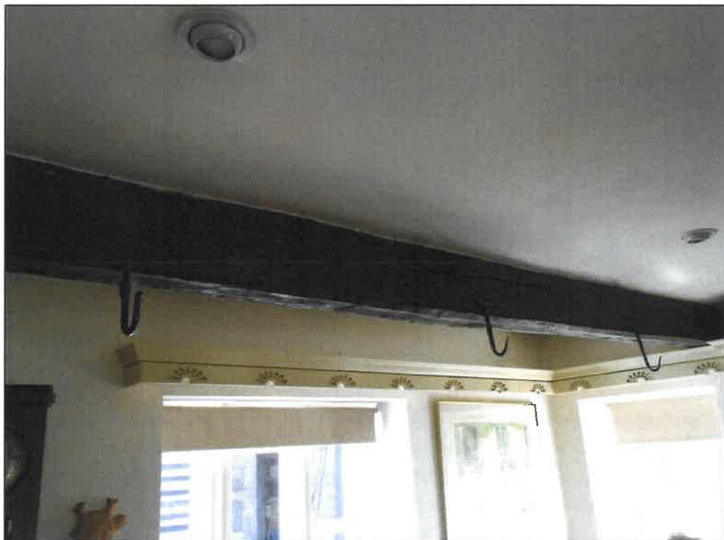
PL15: Hooks present to the underside of a timber beam to the kitchen ceiling.
