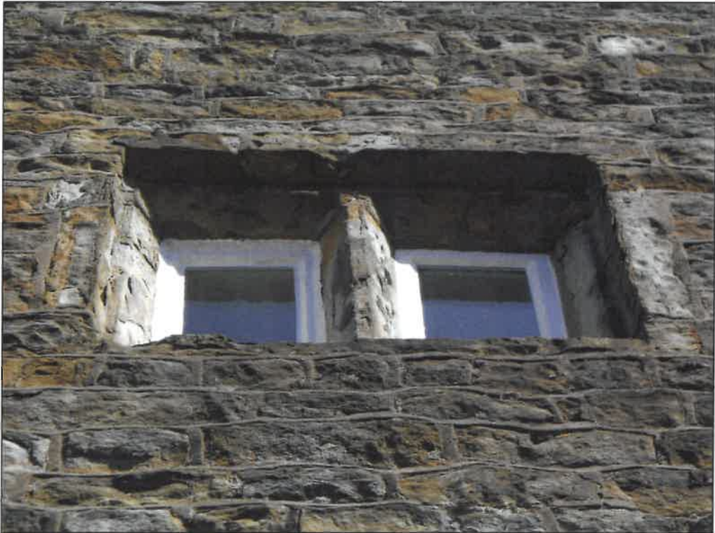
PL10: Window present to the second floor with straight chamfered mullion and jambs.
