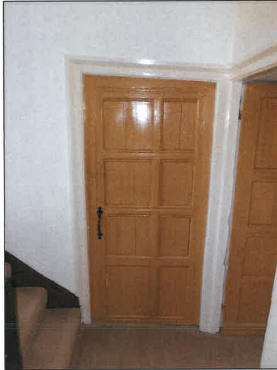
PL12: Original internal door present to the first floor of the building (now fixed shut) to the south east of the building.
