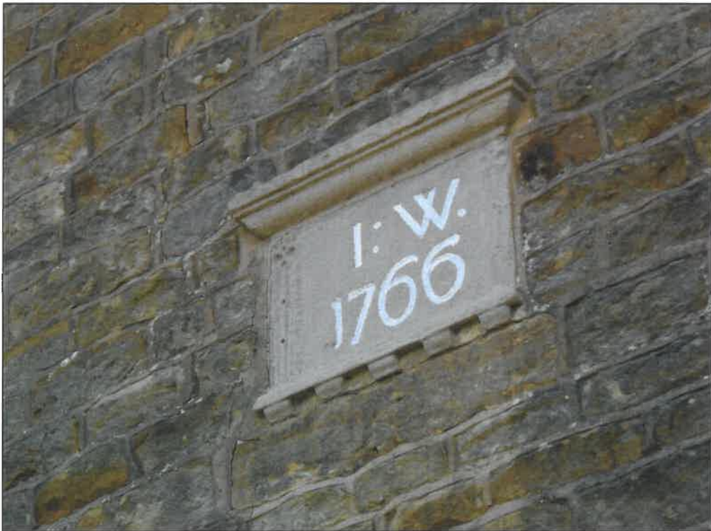
PL07: Date stone present to the front west facing elevation of the building.
