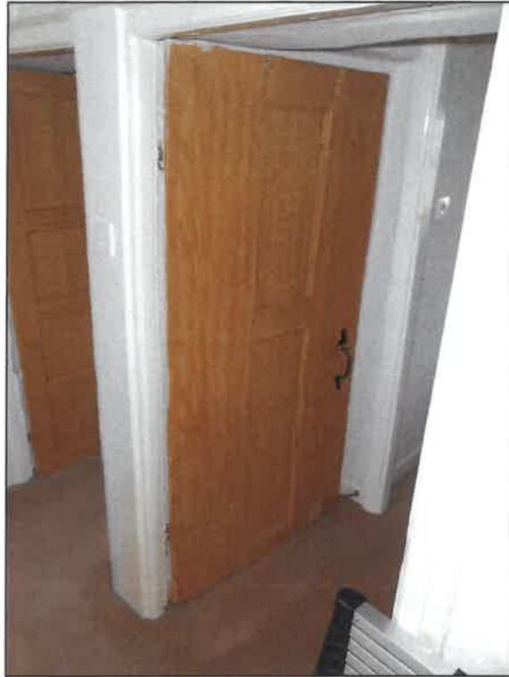
PL14: Original internal door present to the first floor of the building to the front north west bedroom
