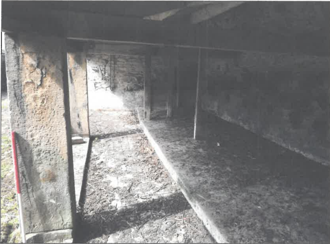
Interior of cart shed, latterly used for stalls, looking south, scale 1m
