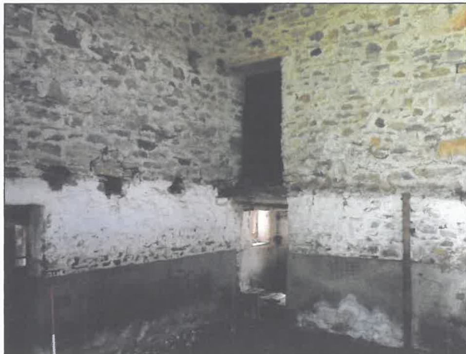
Plate 4. Joist holes and 'tide mark' showing hay loft, looking SE, scale 1m
