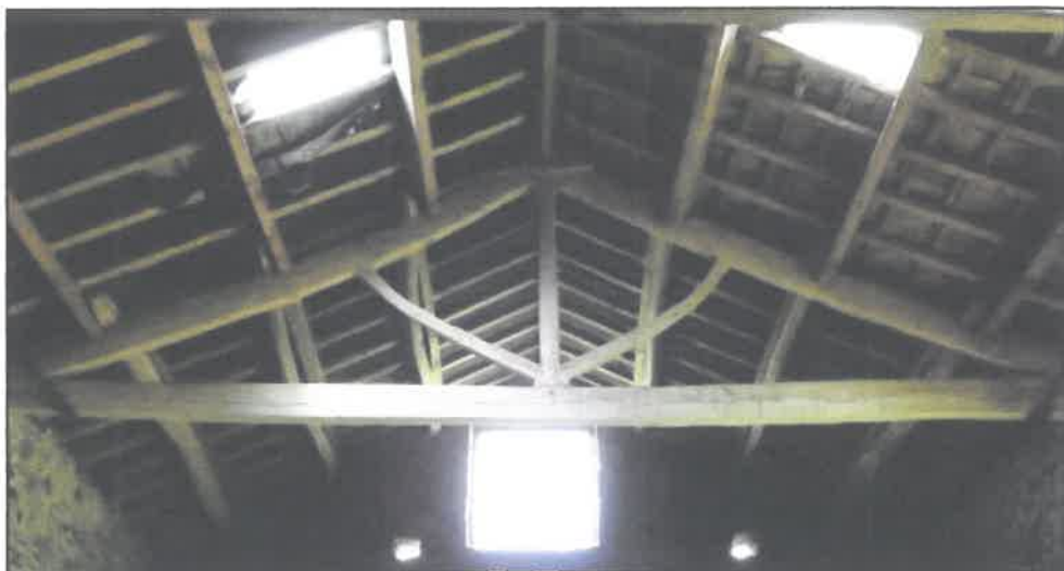
Plate 3. King post truss with curved braces at west end of the barn, looking W
