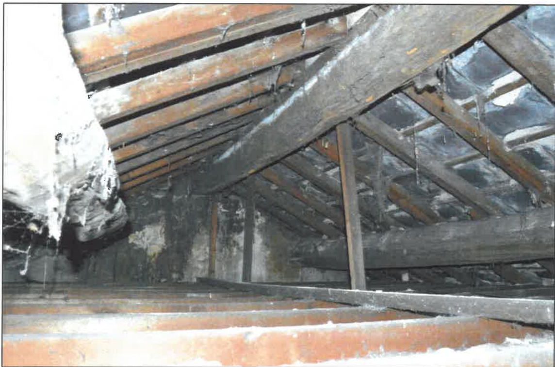
PL14: View of timber roof structure over the south first floor unit of no. 13 Gisburn Road.
