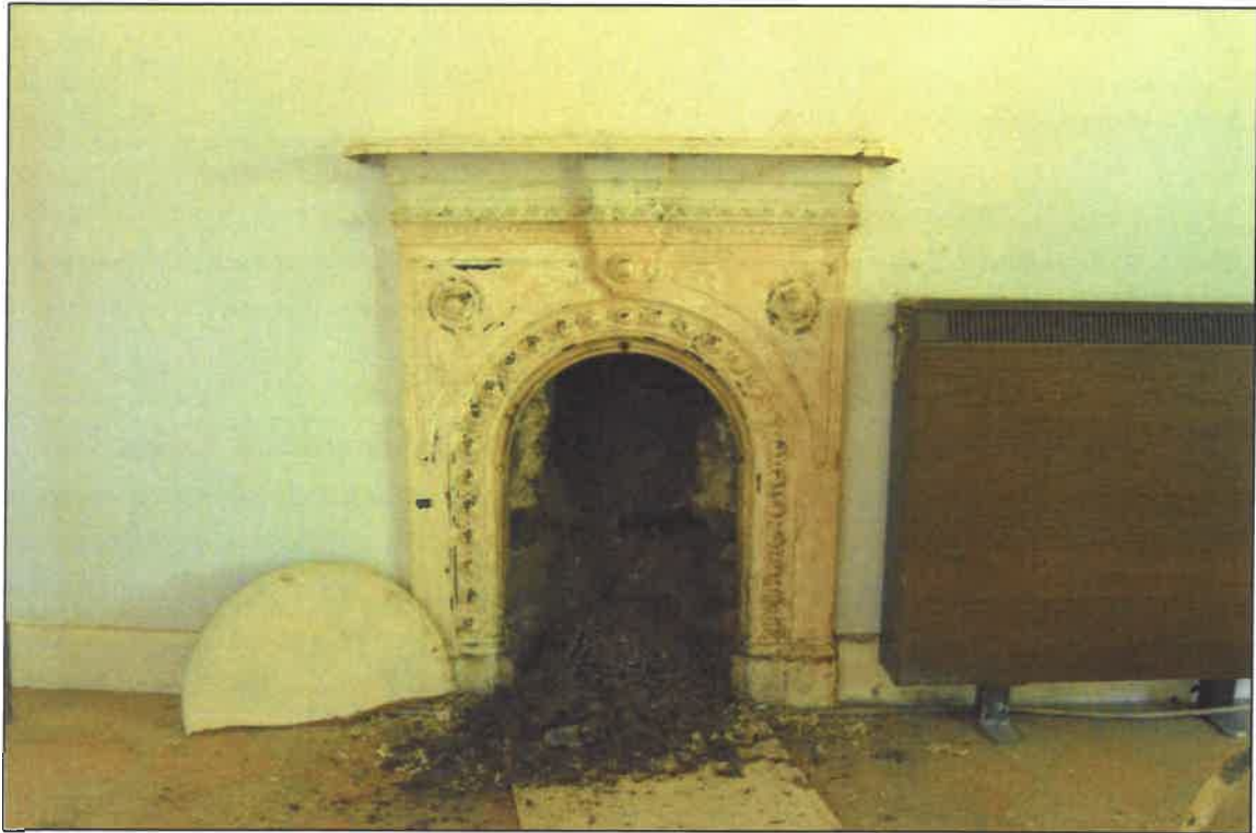
PL13: View of Victorian fireplace within the south first floor unit of no. 13 Gisburn Road.
