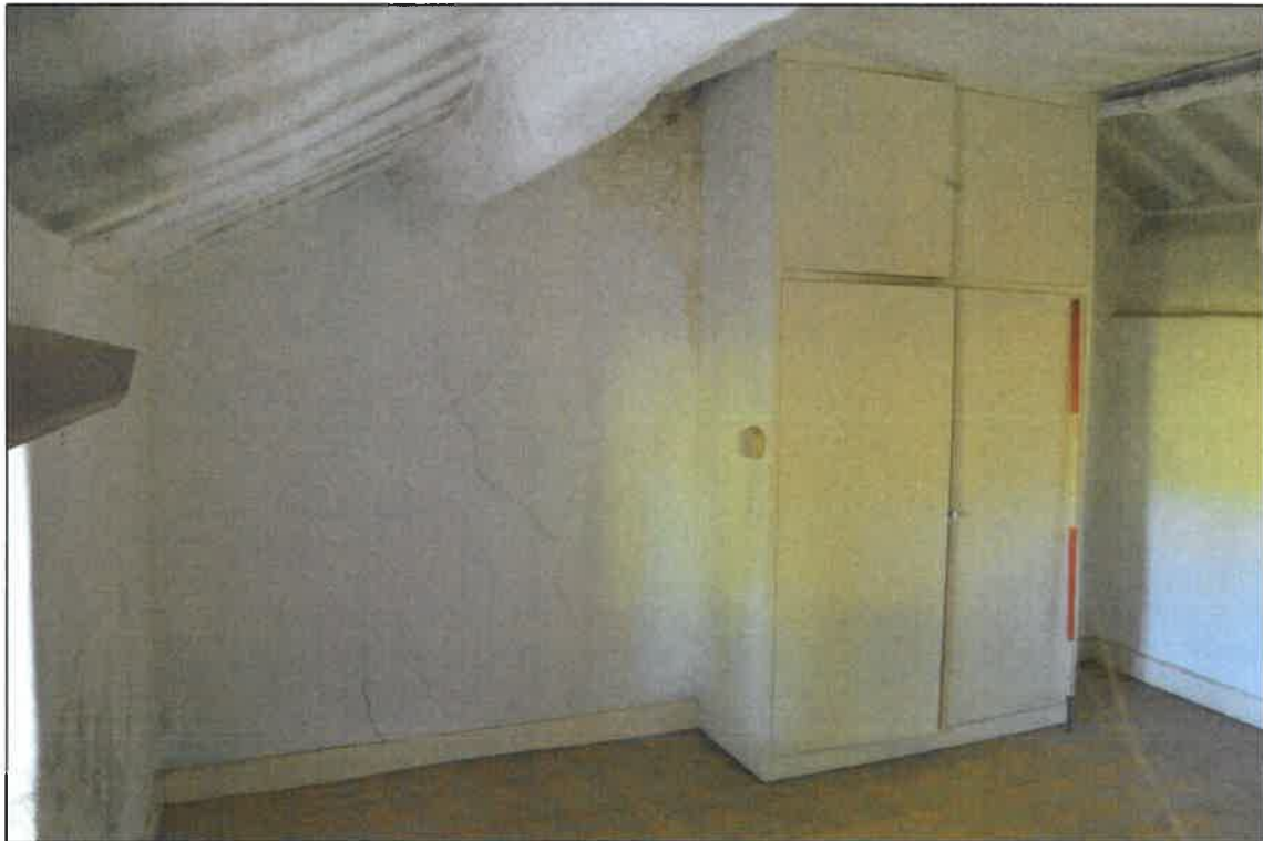
PL11: View west within the first-floor south unit of no.13 Gisburn Road (2m scale).
