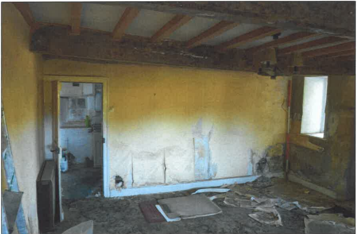
PL05: View north within the ground floor south unit to no.13 Gisburn Road.
