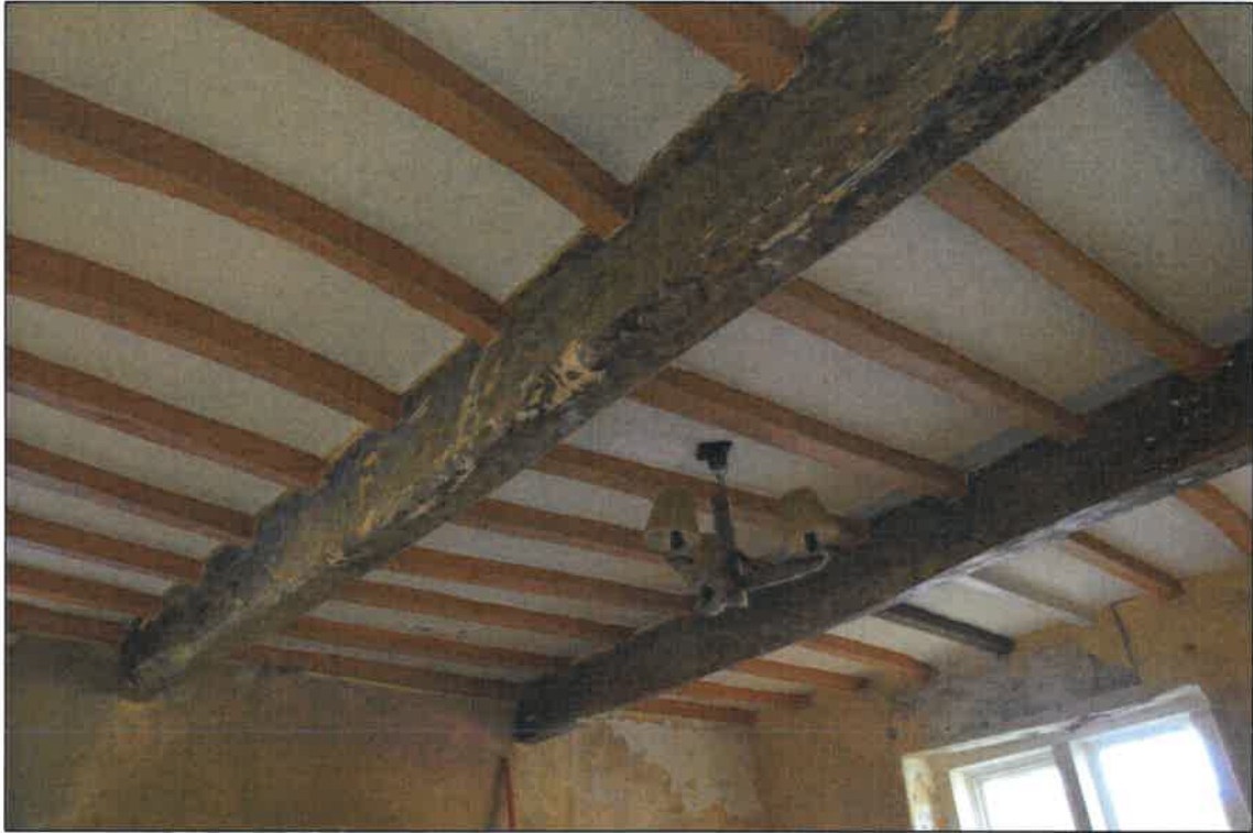
PL06: View of floor structure to the south ground floor unit ceiling to no.13 Gisburn Road.
