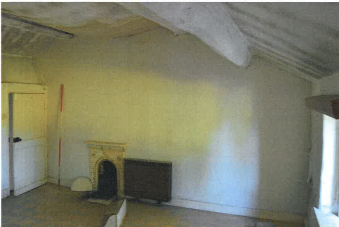
PL12: View east within the first floor south unit of no.13 Gisburn Road (2m scale).
