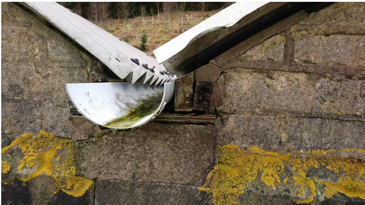
Figure 10: Decaying plywood and timber packing in central gutter
