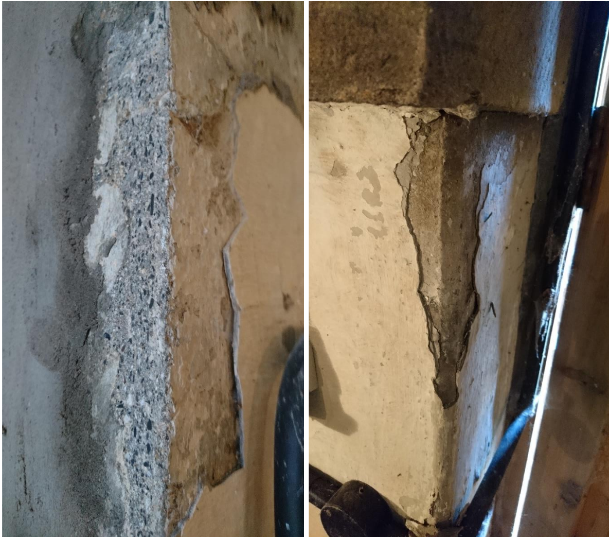
Figure 13: LEFT: Sawn concrete at edge of door opening, RIGHT: Chamfered corner on opposite edge of door opening
