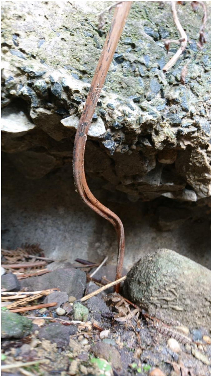
Figure 15: Closeup view of exposed slab with concrete blocks underneath
