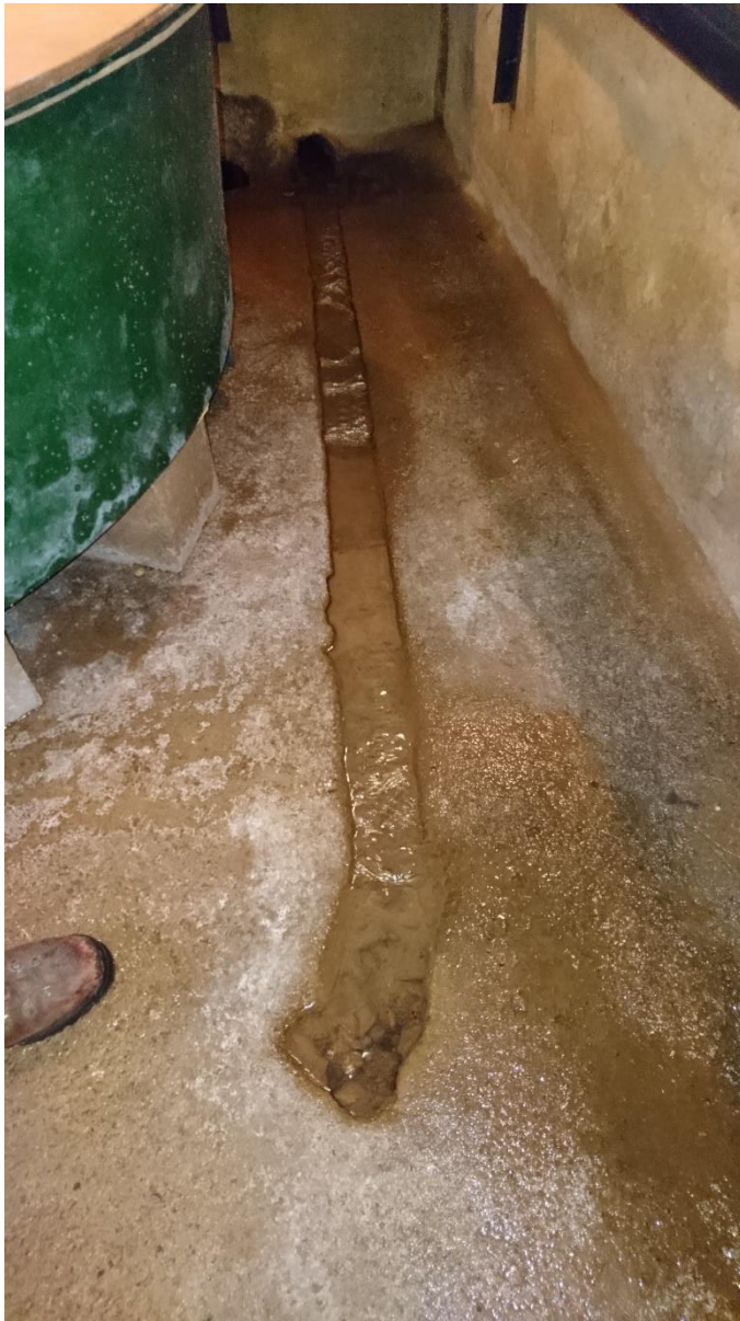
Figure 16: Spring / water issue with cast in channel leading to drain in front wall
