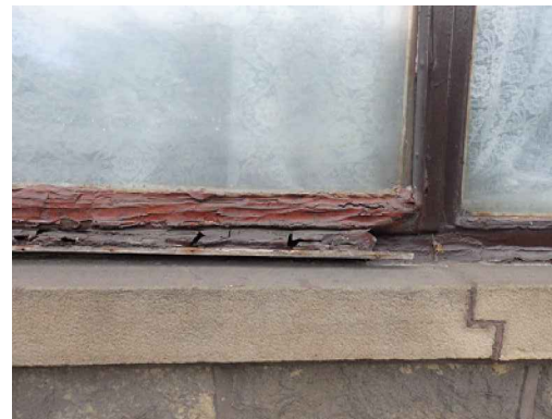
View E - areas of irreparable wet rot to window frame beads
