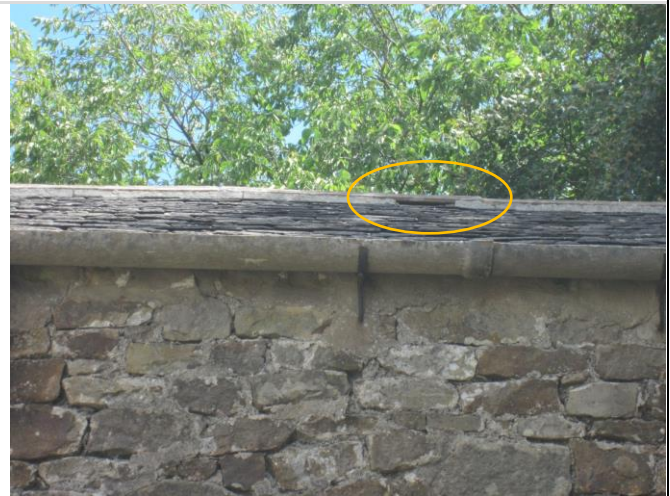
Photo 10: Gaps beneath the ridge copings and between the slates at the detached barn
