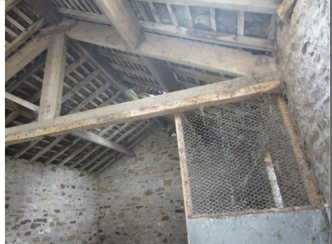
Photo 8: Well pointed internal walls at the first floor of the detached barn
