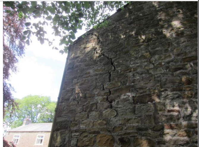
Photo 12: Large crack in the stonework at the southern elevation of the detached barn
