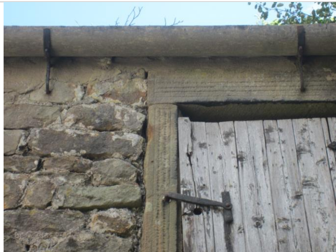
Photo 11: Gaps around the stone window frames at the detached barn
