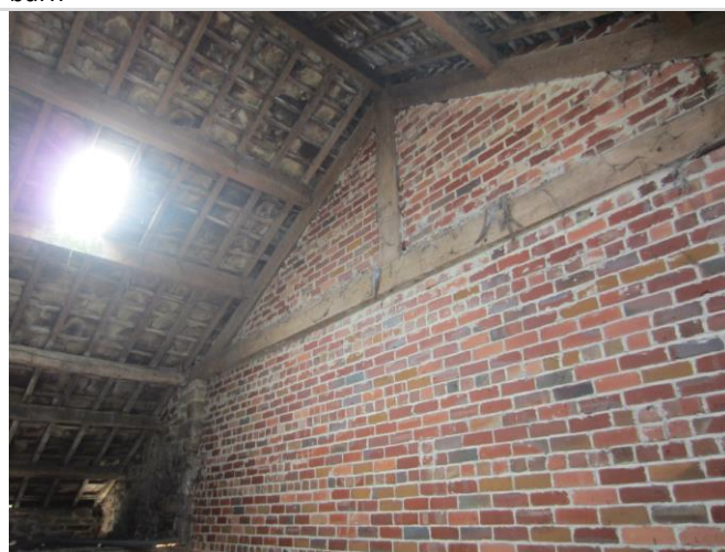
Photo 16: Interior of the attached barn showing the light internal area owing to the presence of skylights (the newer bricks are part of the farmhouse).
