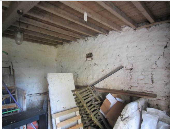
Photo 9: White washed walls at ground level at the detached barn
