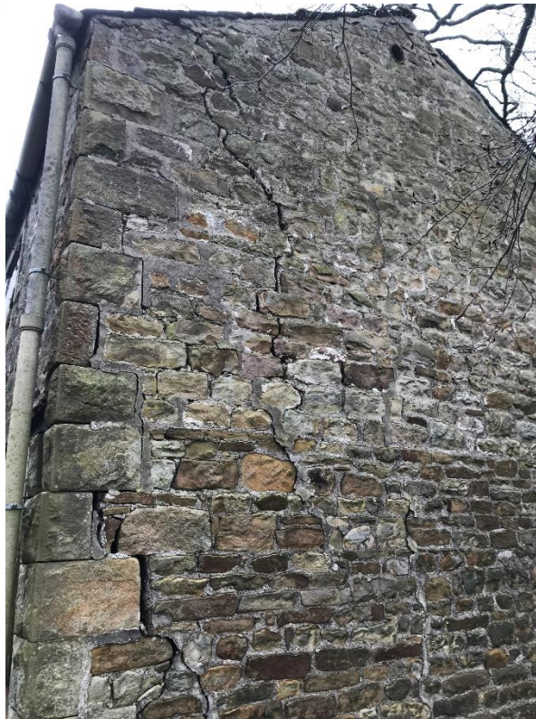
4) Cracking to south gable
