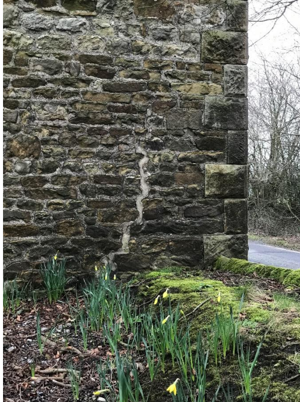
3) Previous crack on south gable, road side
