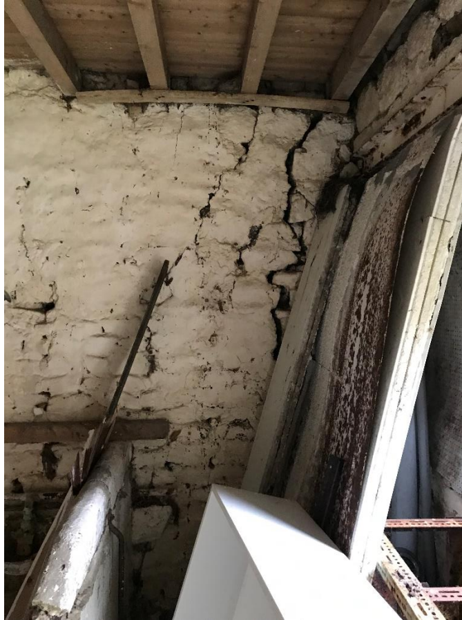
5) Cracking to south gable internally
