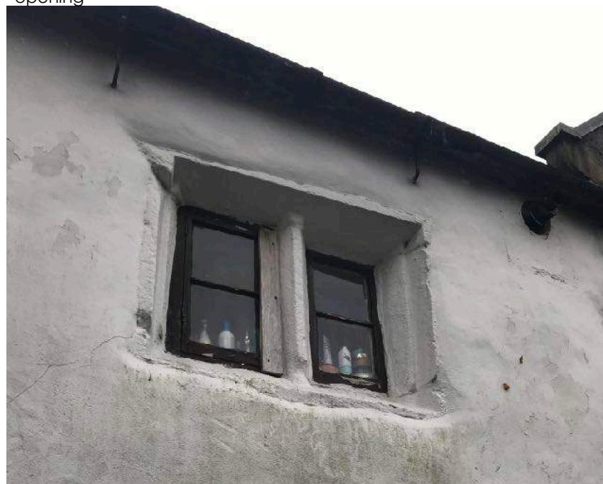
Window 02 : First floor : Original stone surrounds painted with single glazed timber casement frames. 1no. frame fixed shut, 1no. opening.
