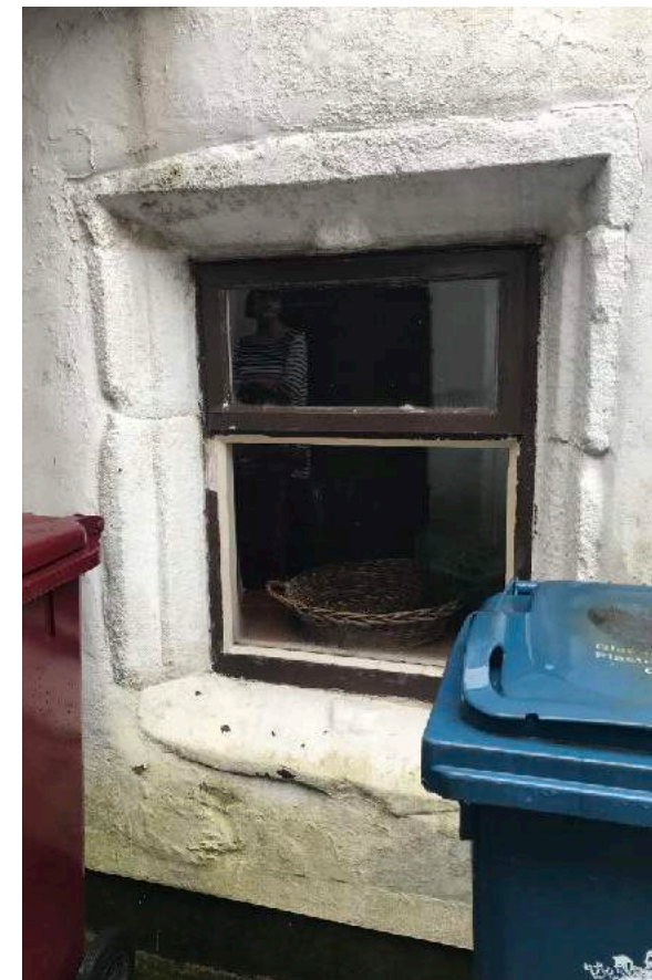
Window 04 : Ground floor : Original stone surround with missing central stone mullion. Single glazed timber casement with top hung opening light
