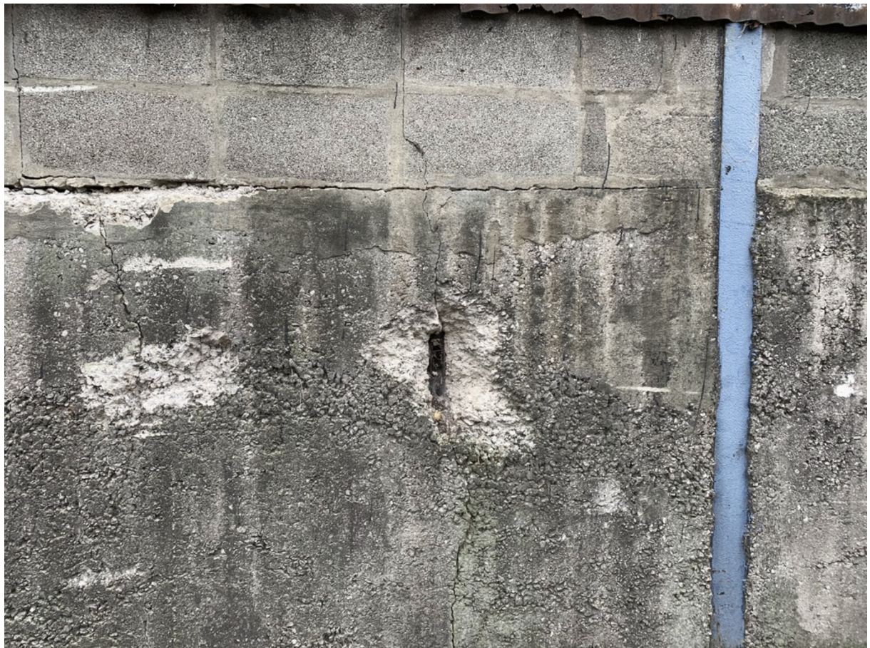
Photo 6 – East Elevation – intermediate column and damage to concrete
