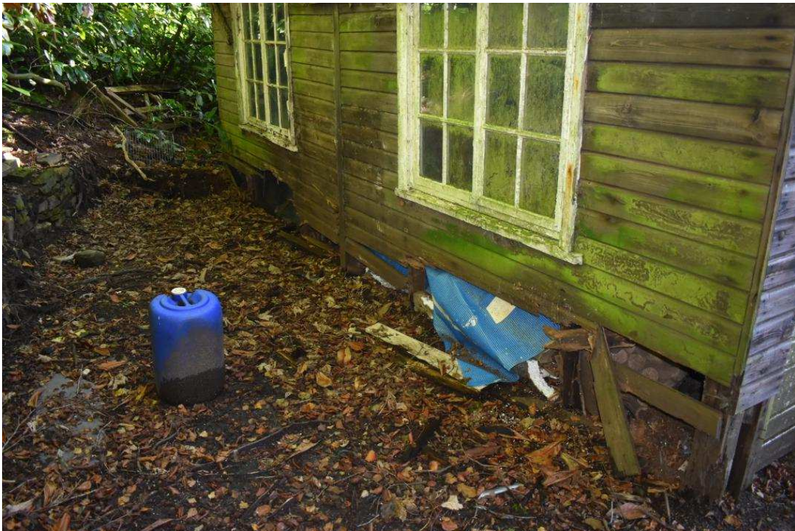
Example of garage disrepair
