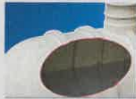
Below Ground Storage Tanks
