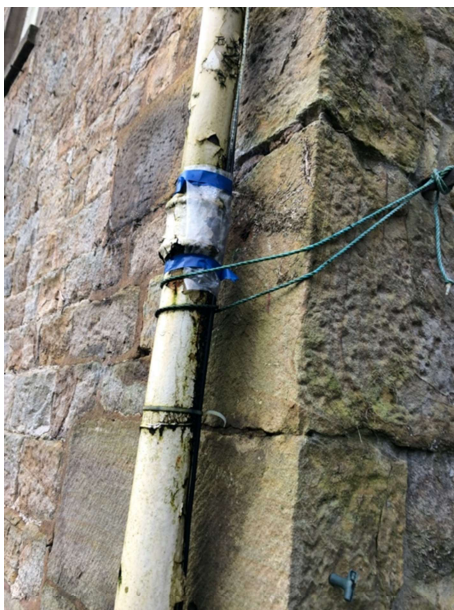
Photo 1 - Corroded cast-iron down-pipe.
