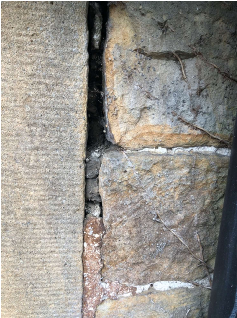
Photo 3 - Lime mortar missing between stones
