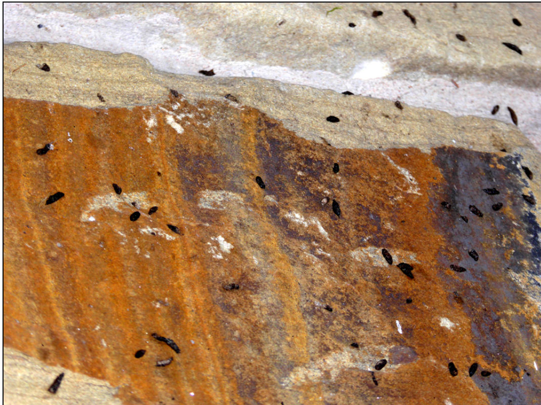
Bat droppings on external wall to north of building. Note that colours are accentuated by rain at time of survey. Image from February 2020
