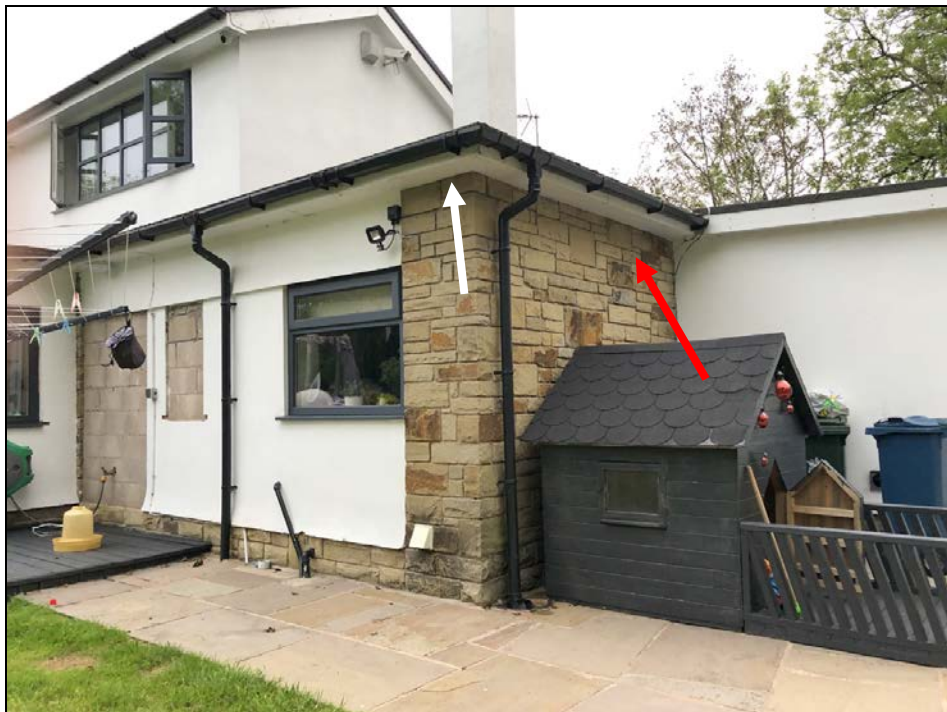
External view of north part of building. Bat emergence point (white arrow) and bat droppings (red arrow). May 2020
