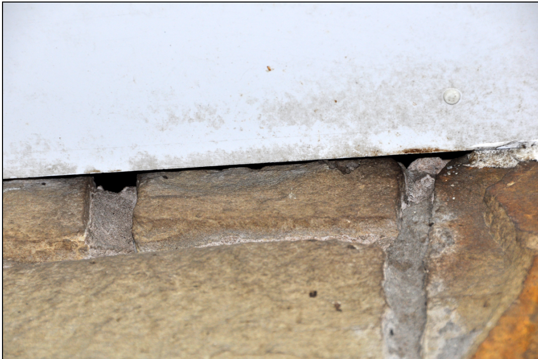
Previous bat access point in north part of building, below soffit edge, showing clear staining from fur oils. May 2020
