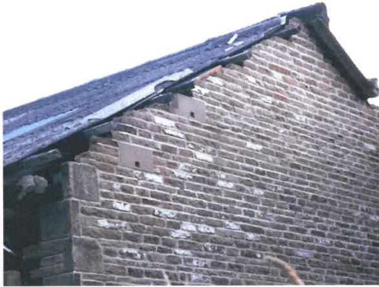
Example of Forticrete boxes in situ
