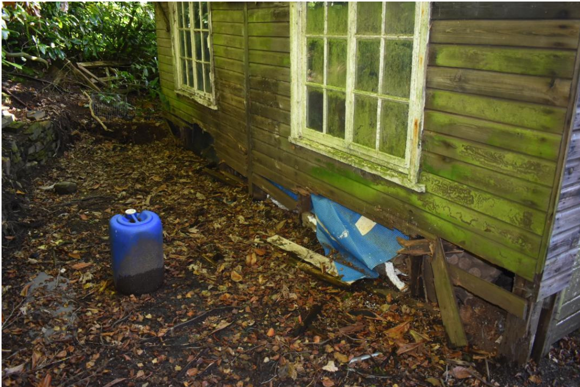
Example of garage disrepair
