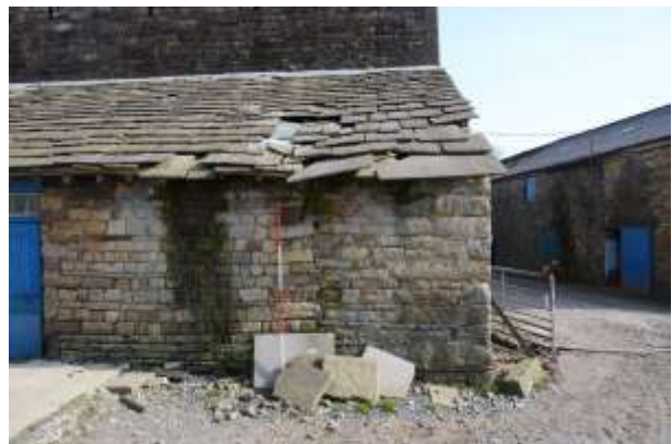
Plate 21 Vertical break in the fabric of the southwest outshut
