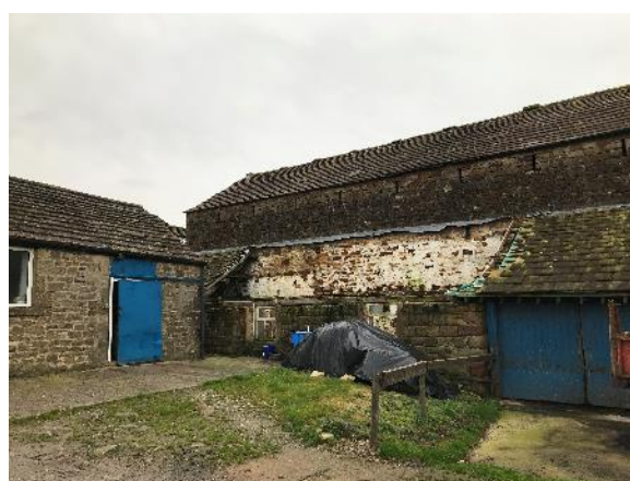
Missing section of lean-to roof to south-west annex
