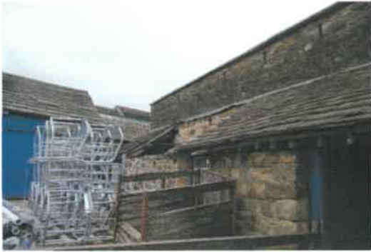
Photo 7 - Dismantled section of roof to south-west lean-to. The lead flashing along the top is loose, creating crevices beneath.
