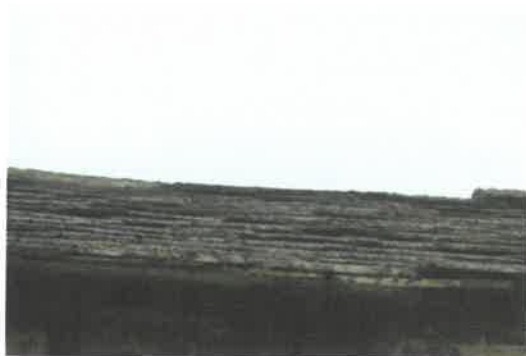
Photo 3 - Raised and loose stone tiles and gaps along the ridge to the main barn roof.
