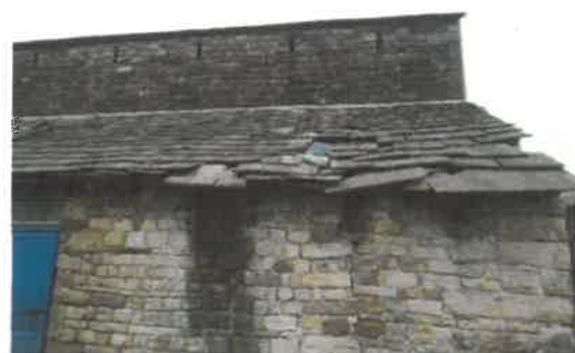
Photo 6 - southern corner of lean-to which is in a poor condition and is beginning to collapse.
