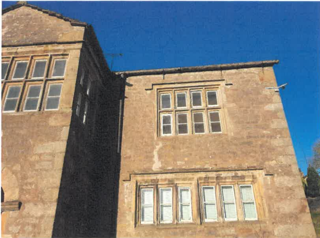
Photo 6: The windows require putty replacement and redecoration on the east elevation
