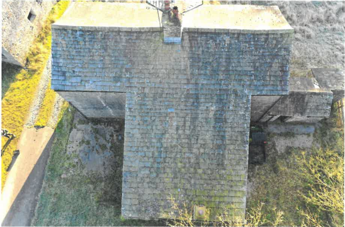
Photo 14: The west slope has quite a large amount of slipped or broken slates
