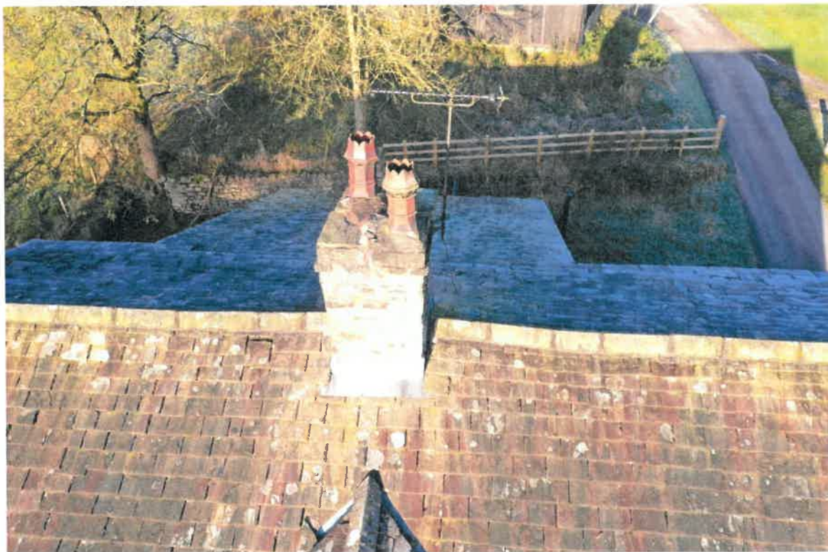
Photo 16: The flaunching on chimney 1 is in a poor condition and requires replacement
