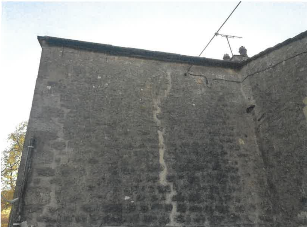
Photo 3: The gutter is damaged, and a large section of downpipe is missing to the west elevation
