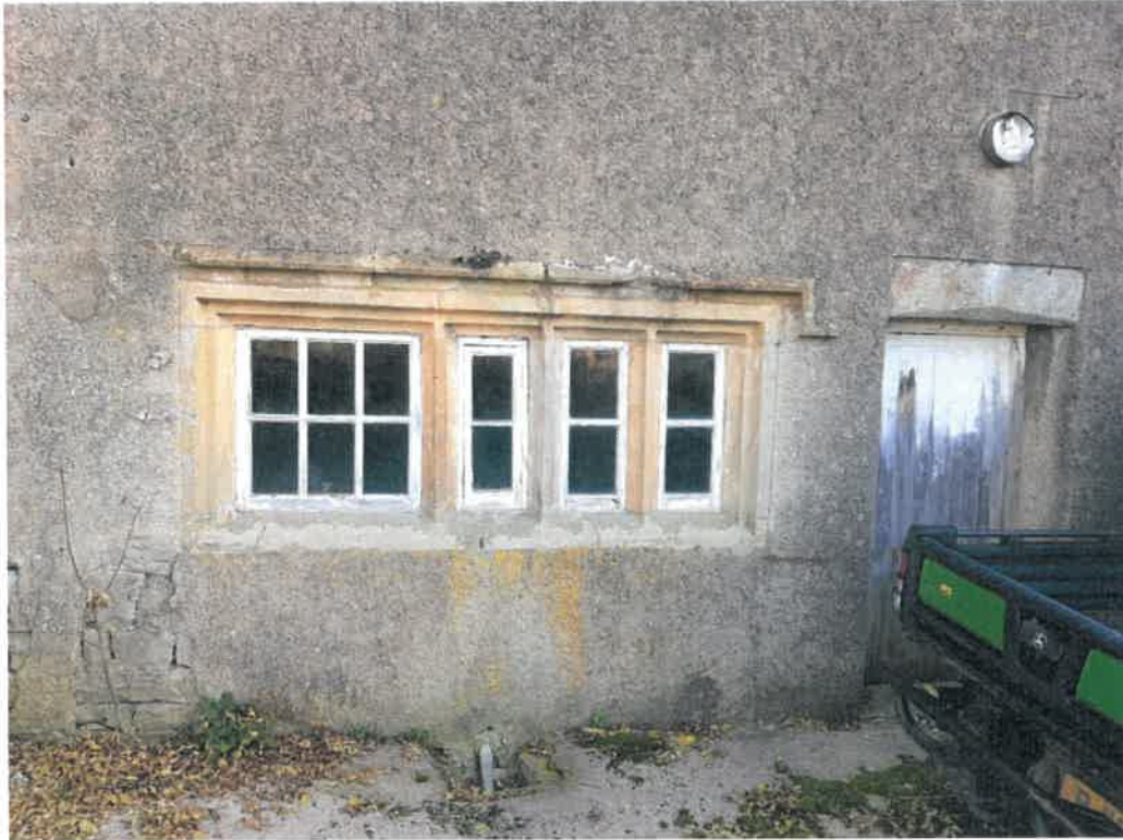
Photo 8: The windows to the south elevation require putty replacement and decoration. The timber door also requires redecoration.
