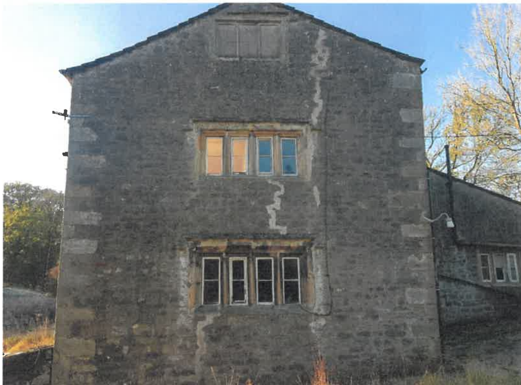
Photo 7: There is one missing window that requires replacement and one window that requires reglazing, the remaining windows require putty replacement and decoration on the north elevation
