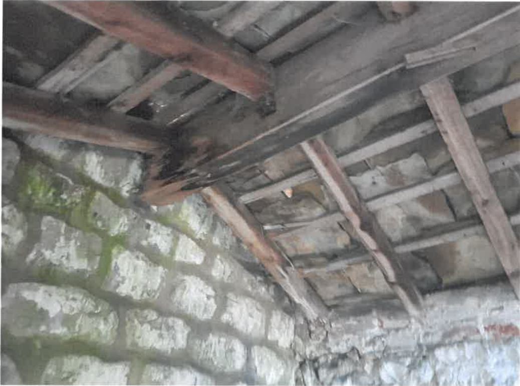
Photo 10: The ridge beam is rotten at the bearing end and will require a splice repair
