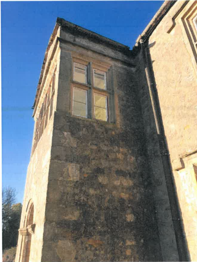
Photo 1: There are sections of the gutter missing on the east elevation
