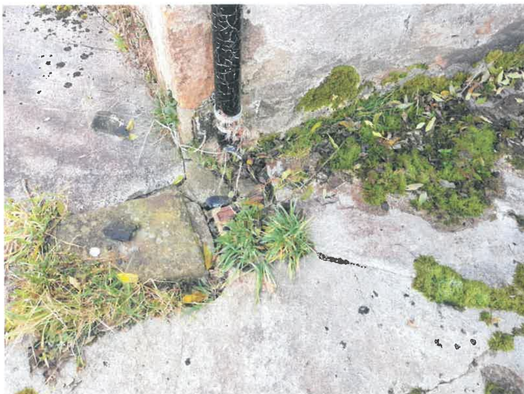
Photo 13: The gullies are blocked and require clearing and jetting
