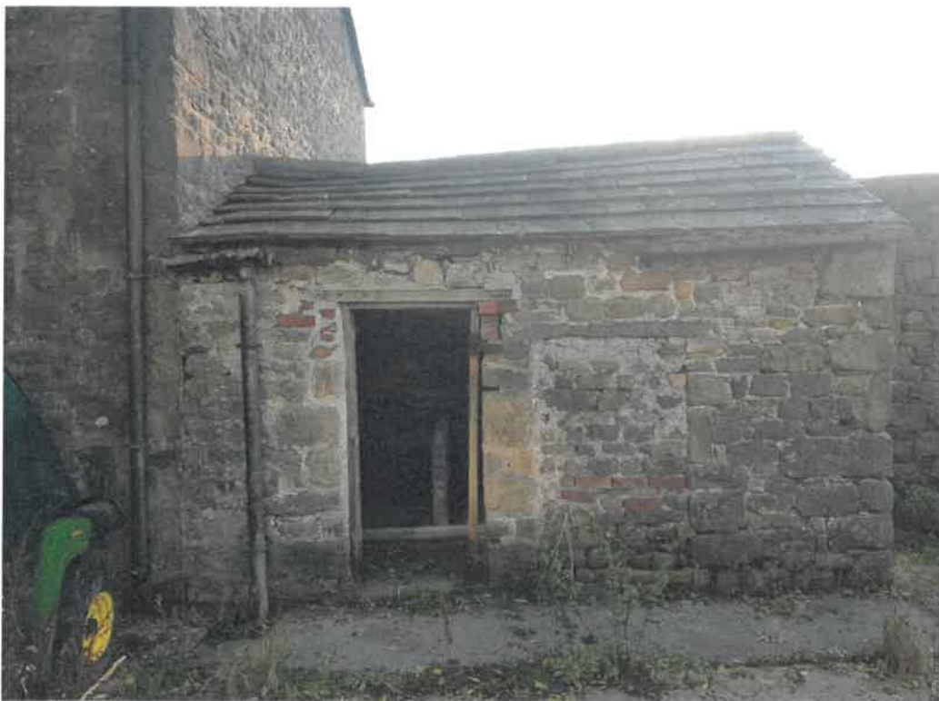
Photo 11: The roof has sunk as a consequence of the rotten ridge beam
