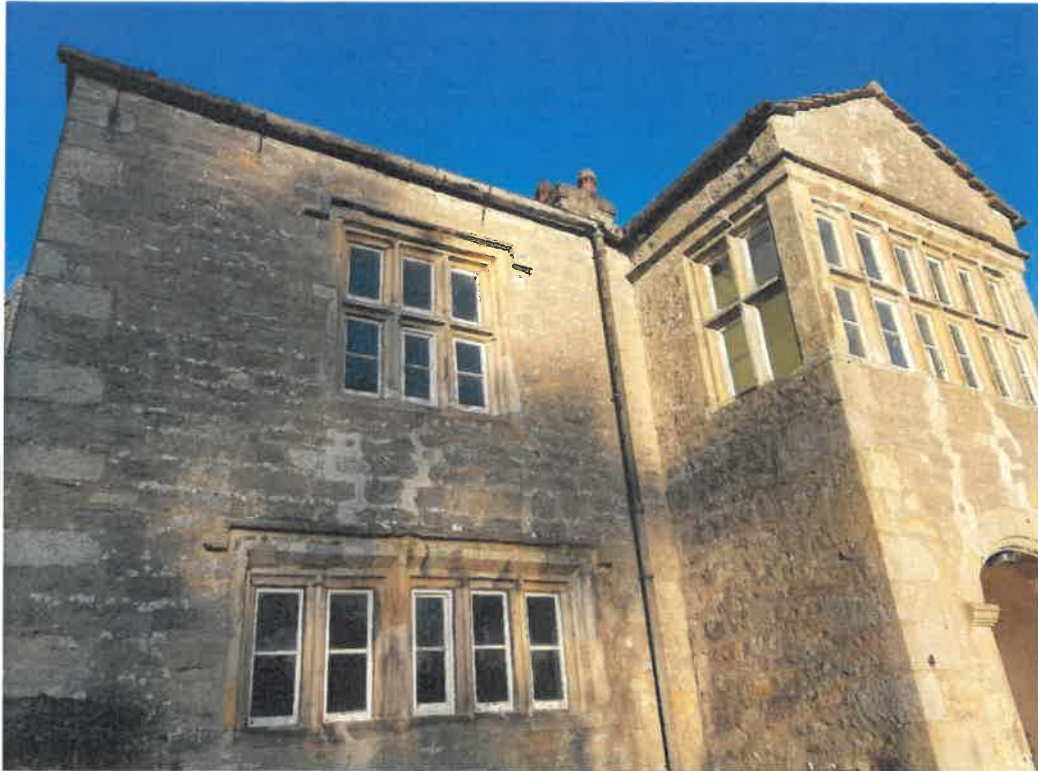
Photo 2: The gutter is damaged and there are multiple splits in the downpipe on the east elevation
