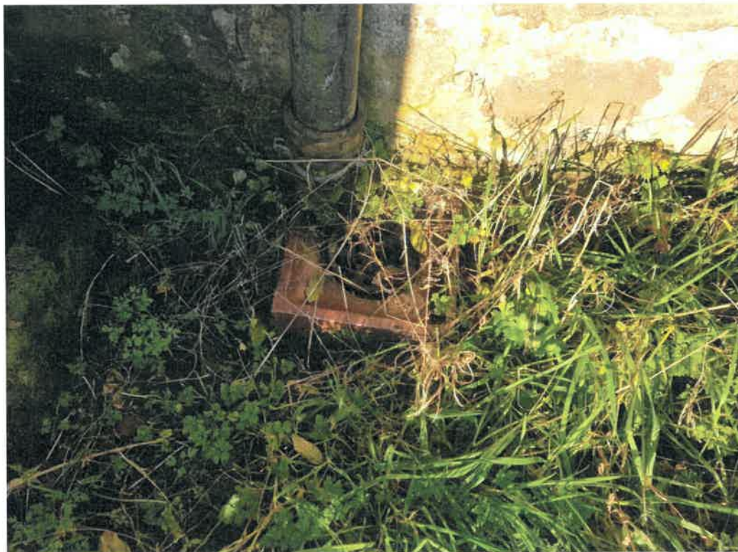
Photo 12: The gullies are blocked and require clearing and jetting
