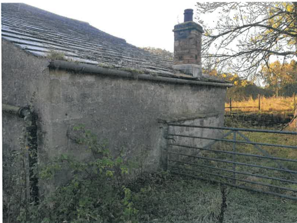
Photo 4: The plastic gutter has no outlet and is full of vegetation to the west elevation
