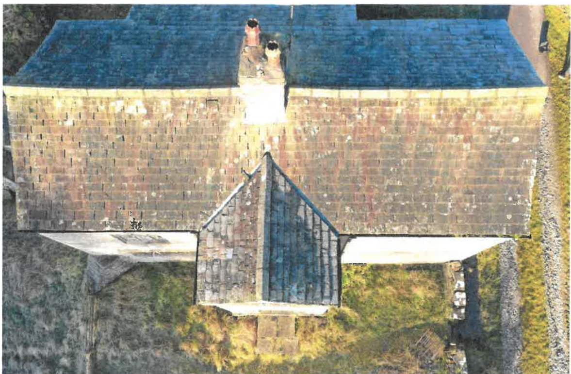
Photo 15: The east slope and main entrance slopes have a small amount of slipped or broken slates
