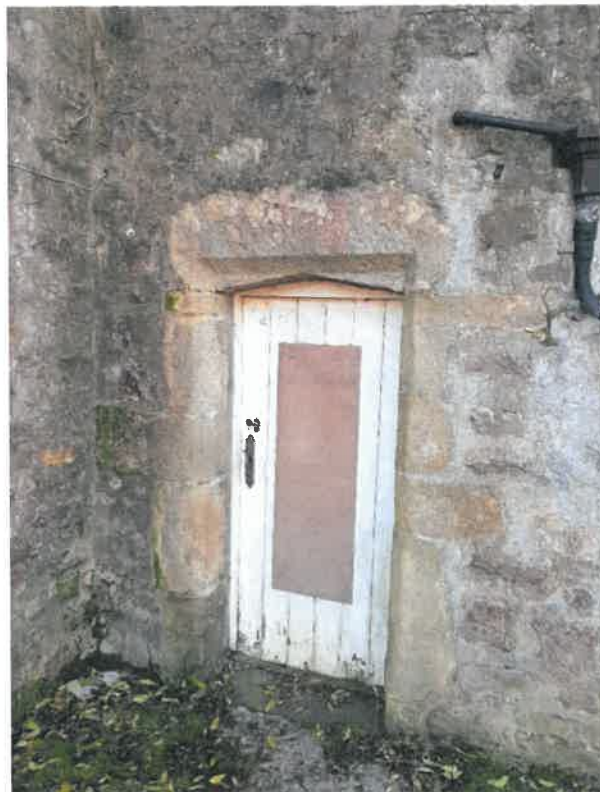
Photo 9: The timber door is covered with plywood boarding and requires repair and decoration
