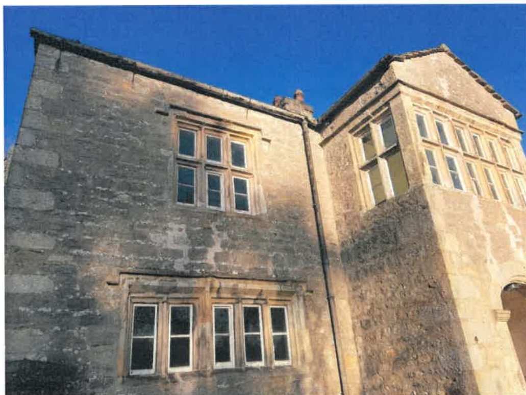
Photo 5: There is one missing window that requires replacement, the remaining windows require putty replacement and decoration on the east elevation
