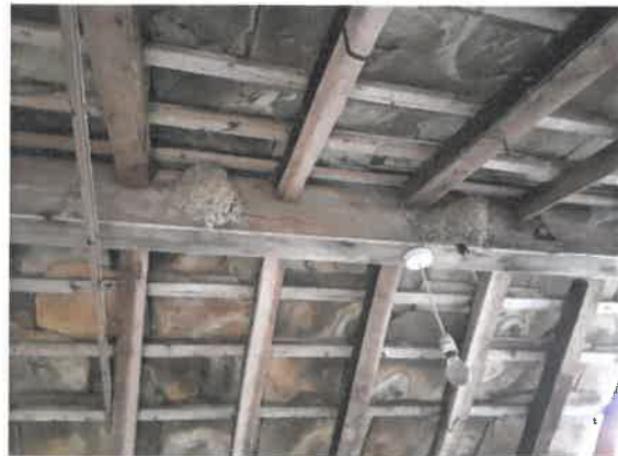
Photograph 12: Unlined roof and swallow nests within the outbuilding.
