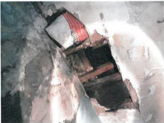
Photograph 7: Hole in the ceiling located above the Aga.
