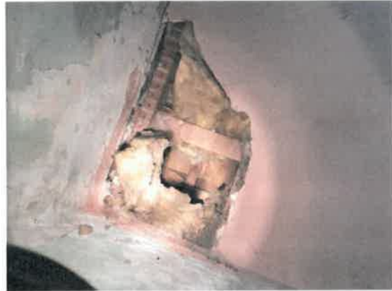
Photograph 8: Hole in the ceiling located within the south-eastern bedroom.
