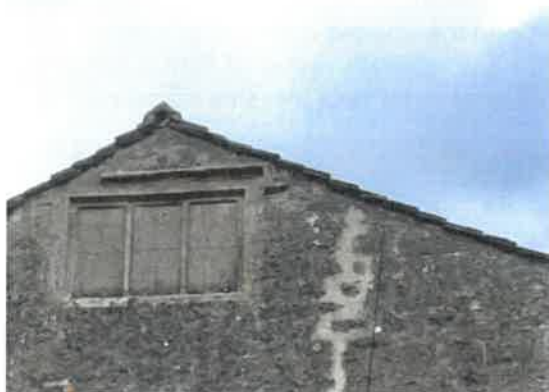
Photograph 5: Gaps beneath the ridge tile and edge tiles on the north-eastern gable end.
