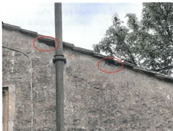
Photograph 3: Areas of missing mortar (circled) along the roof verge on the northern elevation of the catslide roof.
