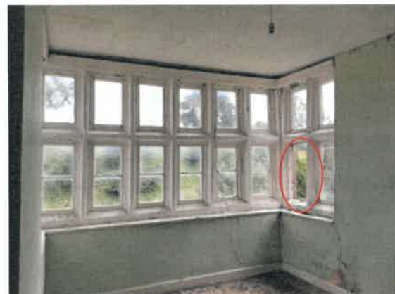
Photograph 4: Missing window pane in the bay window.
