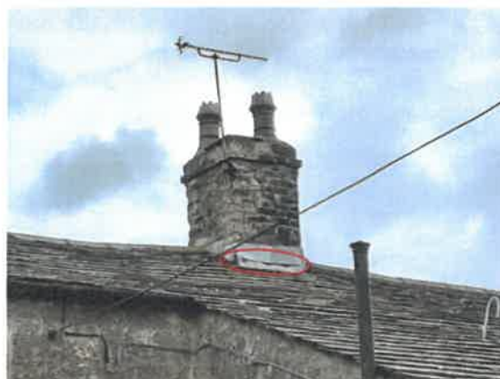
Photograph 6: Areas of lifted lead flashing on the main chimney (circled).
