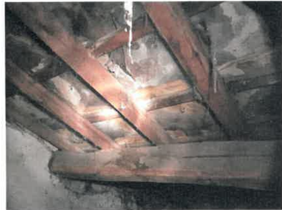
Photograph 10: Unlined roof present within the loft space located off the bathroom.
