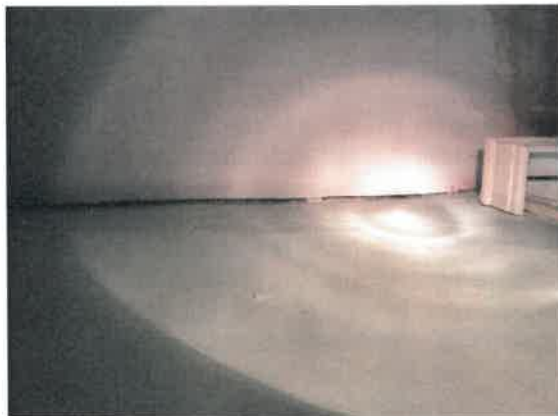
Photograph 9: Narrow crevice between the external wall plate and the ceiling within the south-eastern bedroom.
