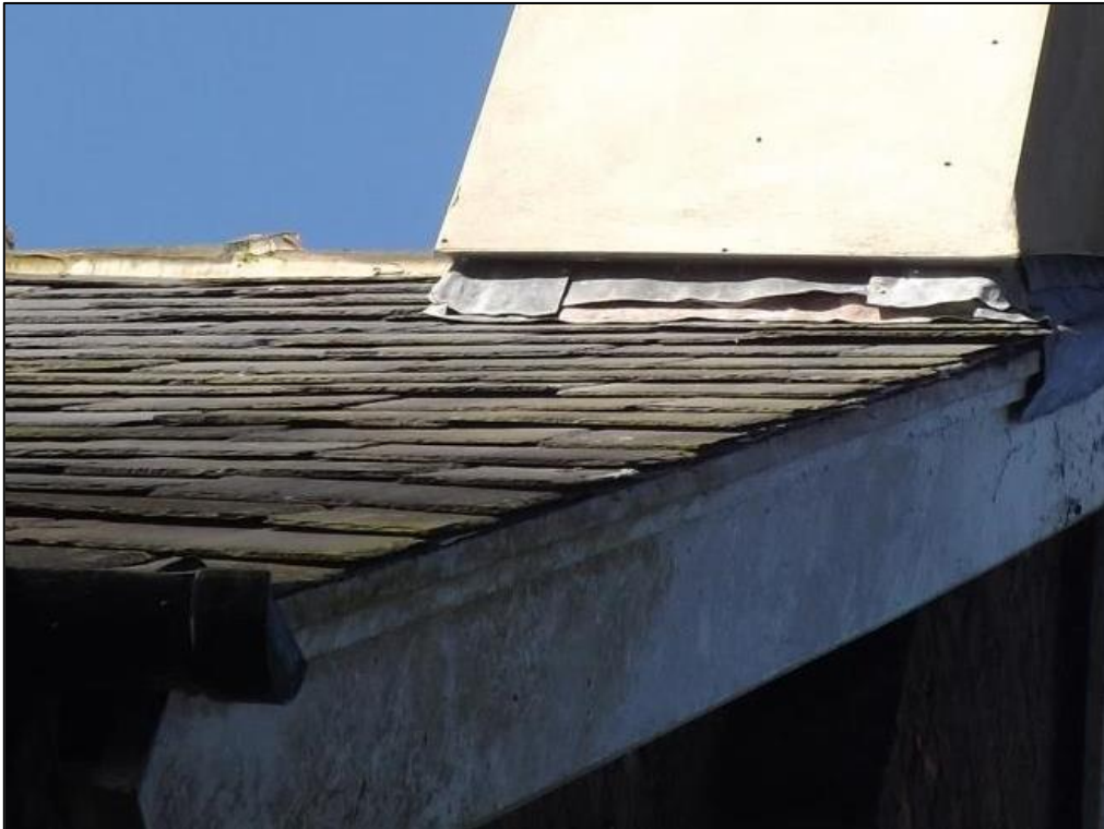
Plate 2: Multiple gaps were visible beneath the roof tiles of the building and around the lead flashing surrounding the chimney. Bat droppings were also visibly adhered to the chimney breast.
