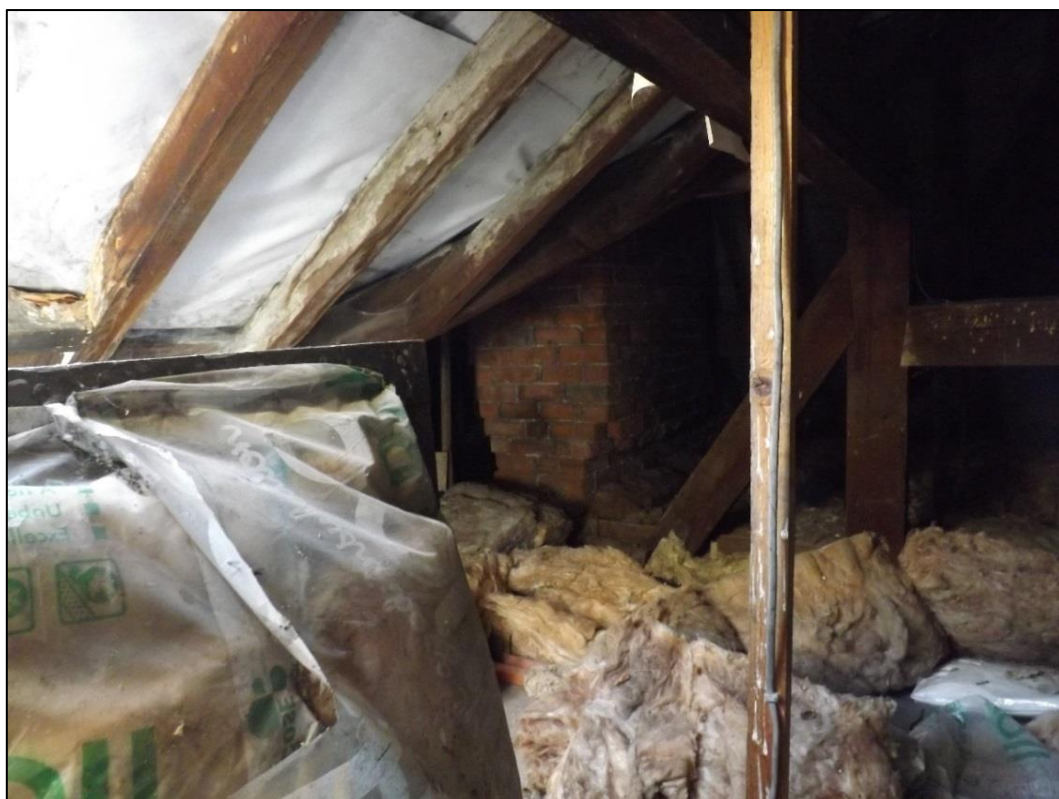
Plate 11: Some gaps were present in areas of the roofing membrane.
