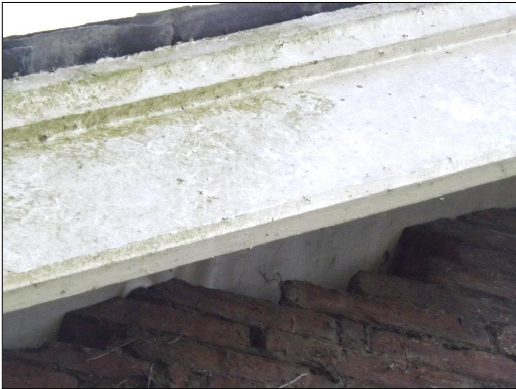
Plate 4: The brickwork along the wall plate was not tightly fitted and contained a number of gaps suitable for bats to utilise.
