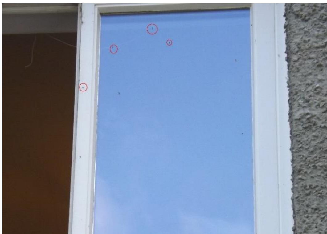
Plate 6: Bat droppings present upon windowpanes on the building.
