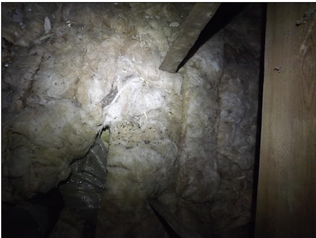
Plate 8: Clusters of bat droppings were present in areas throughout the loft.
