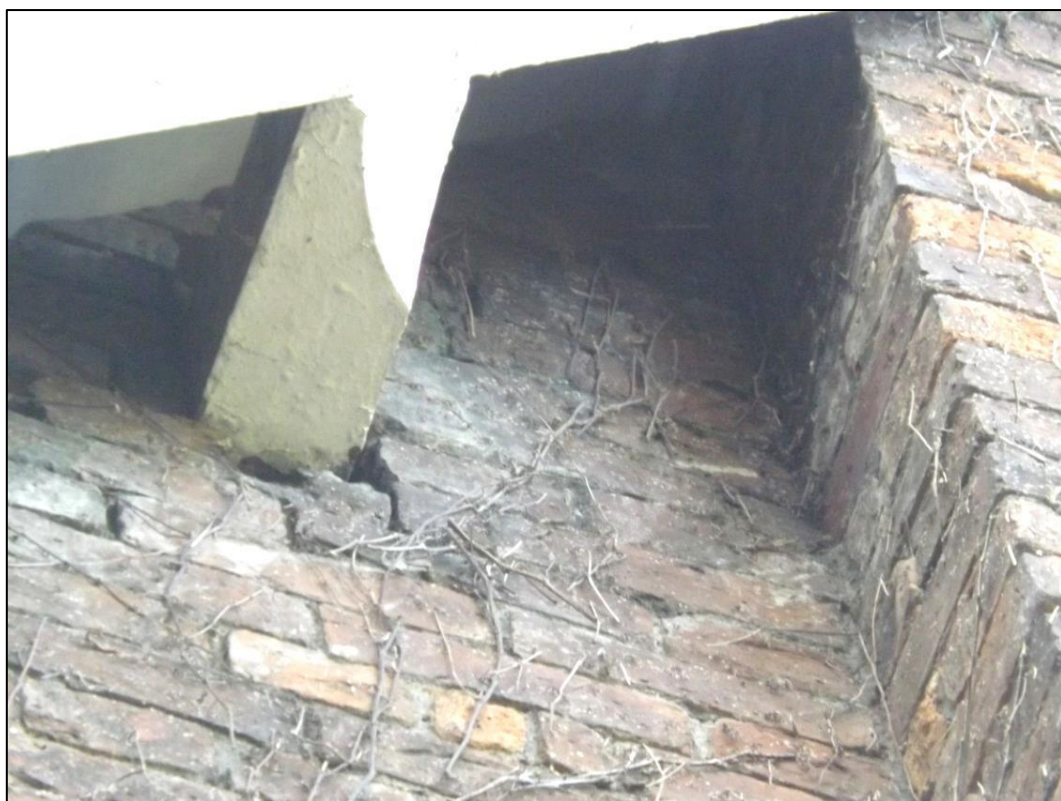
Plate 5: Gaps were also present in the brickwork around roof purlins.
