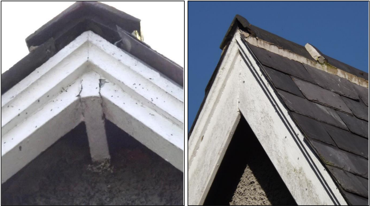
Plate 3: Numerous bat droppings were observed on fascia boards beneath the gable end ridge tiles.
