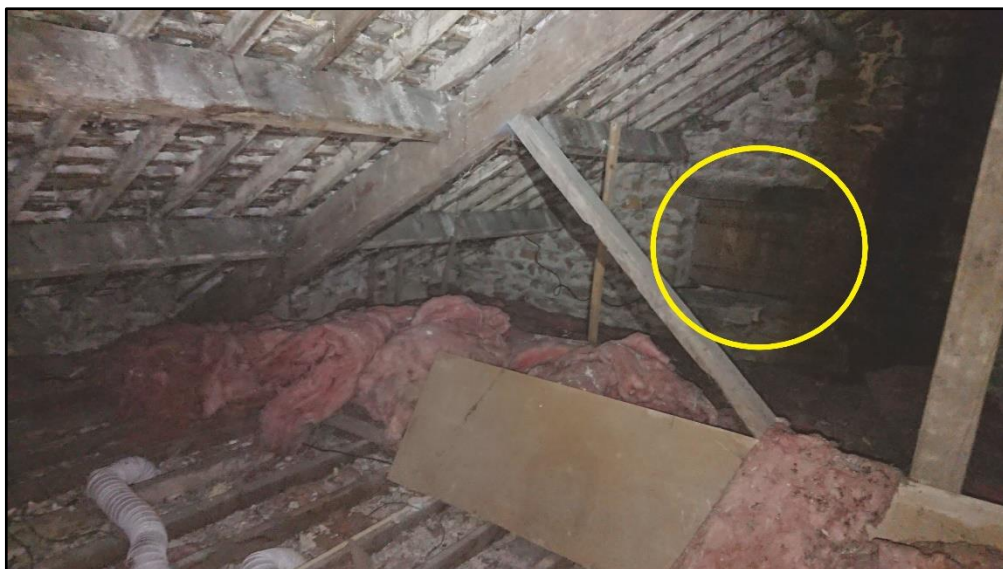
Figure 22. Loft void in main house, with access to next void to the west marked.
