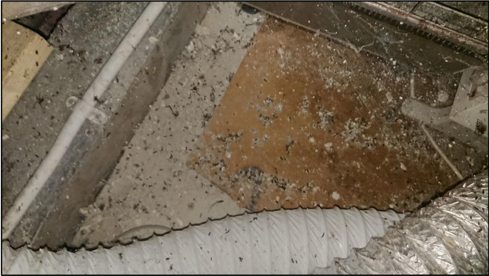
Figure 20. Bat droppings scattered in centre of main loft void.
