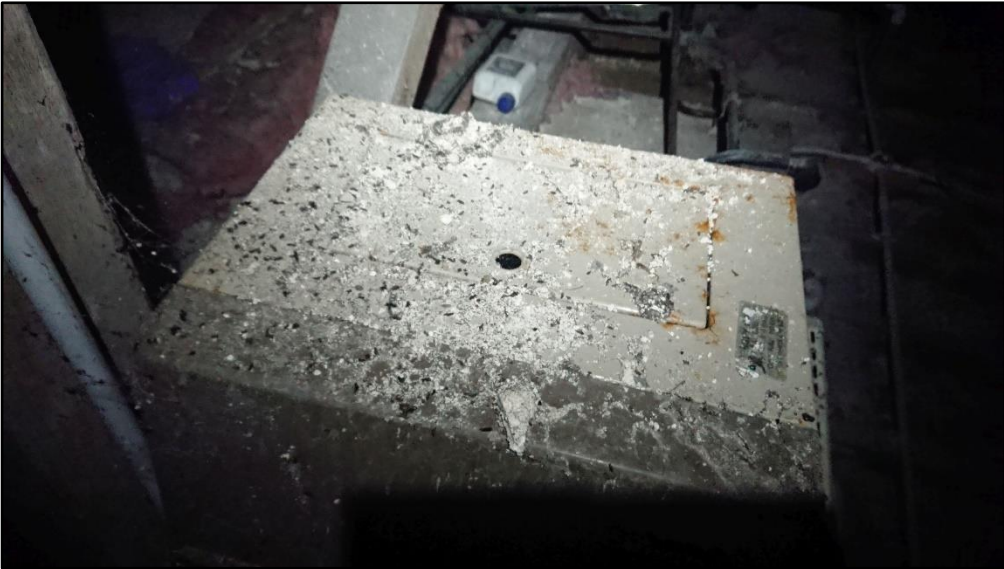
Figure 19. Bat droppings scattered in centre of main loft void.
