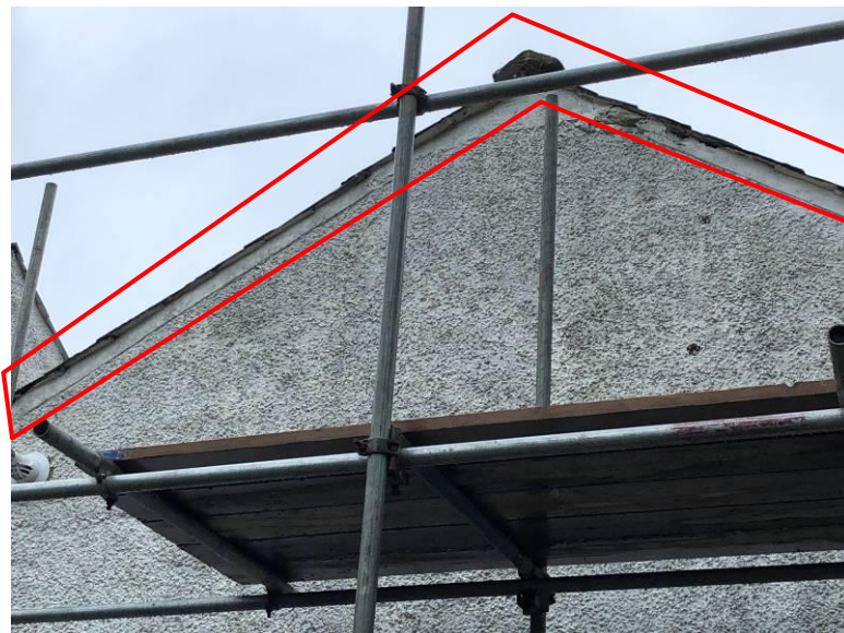
Plate 4: Gaps at roof verge of the house indicative
