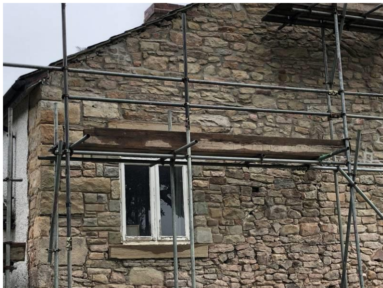
Plate 6: Abundant crevices in stonework and at roof verge indicative
