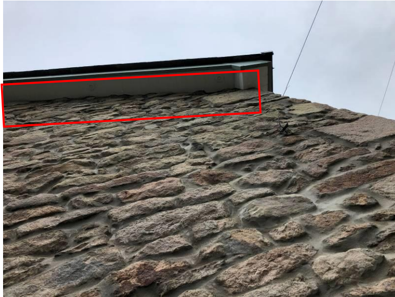
Plate 5: Gaps beneath newly fitted UPVC soffit indicative
