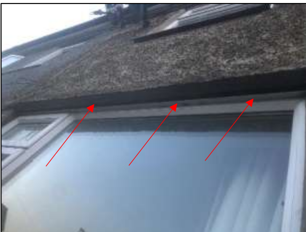
Photo 3: Gap along the lintel above the ground floor window
