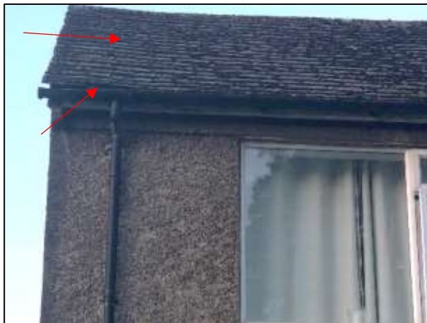
Photo 5: Southwest corner of west elevation – lifted or dropped tiles with gaps.
