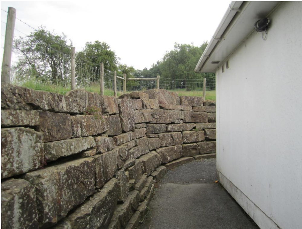
2 Retaining wall at the rear of the site giving context to the change in levels.
