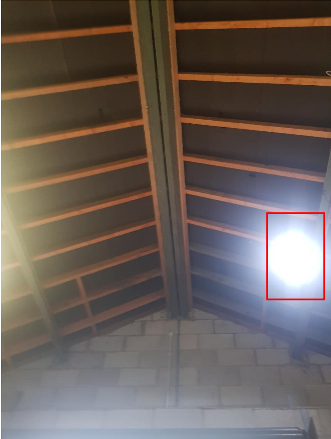
Image 5. Hole in roof of B1, highlighted red.
