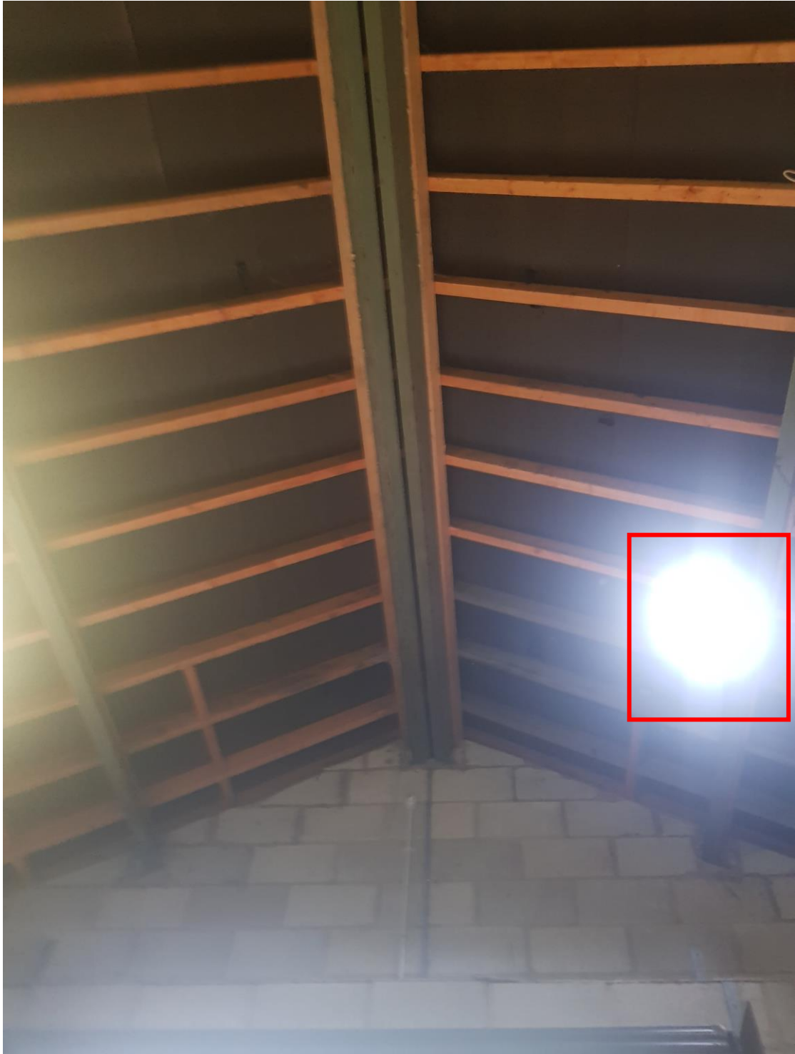
Image 5. Hole in roof of B1, highlighted red.
