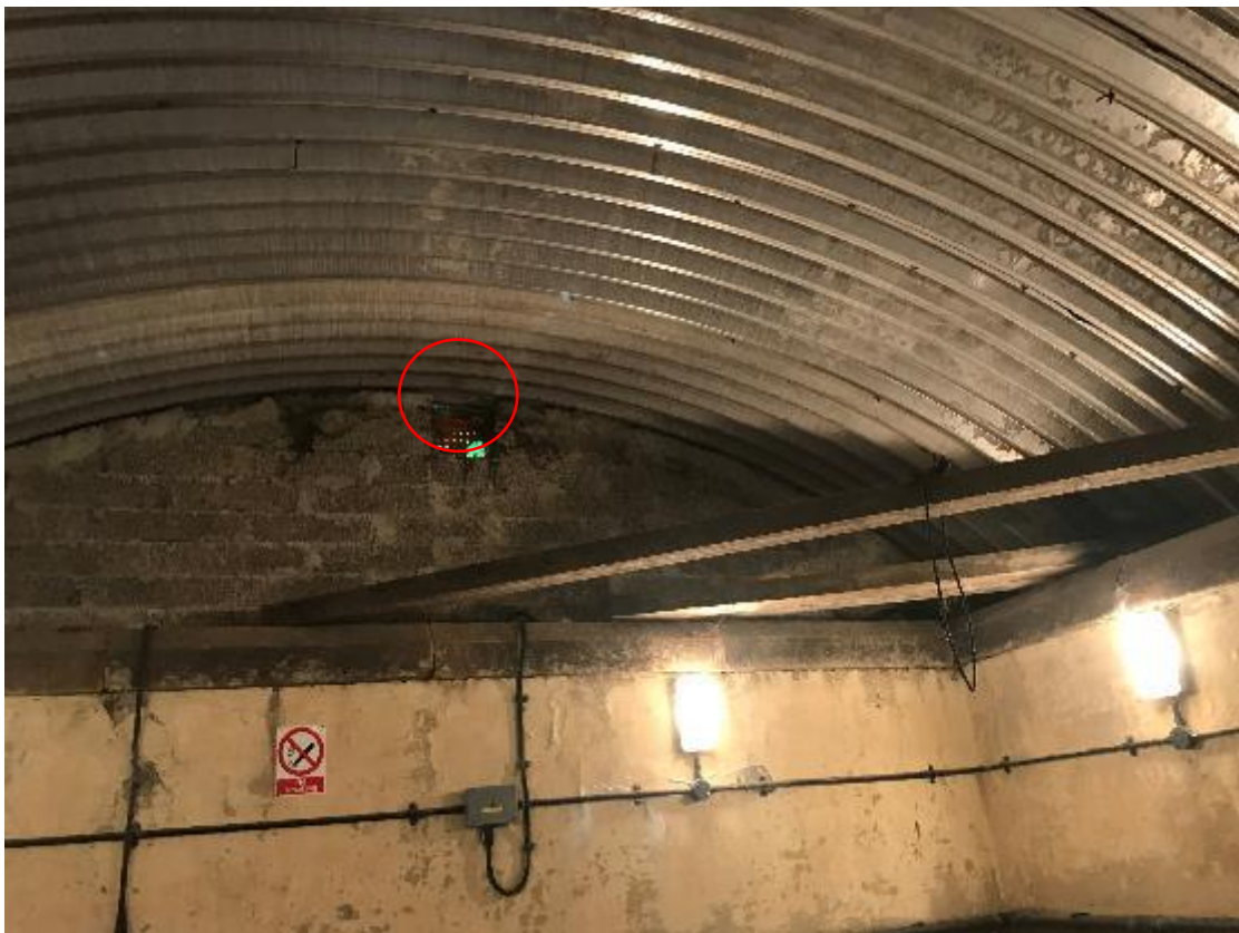
Image 8. Gap in air brick in B2
