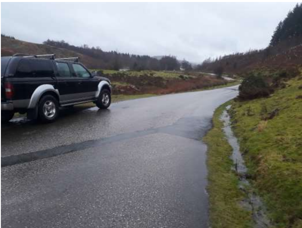
Hard shoulder at north side of bend at (pin no.6)
