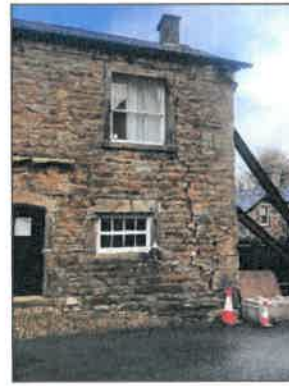
Photo 6: External crack on southern wall of 1.
