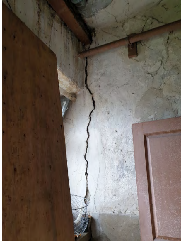
Figure 21 View of crack in ground-floor WC/storeroom
