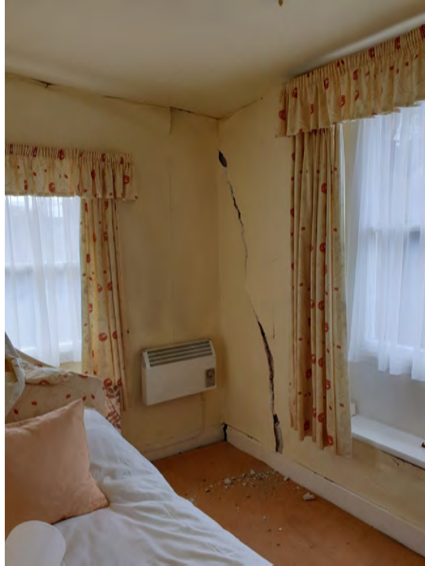
Figure 17 View of crack along south-eastern wall at first-floor level
