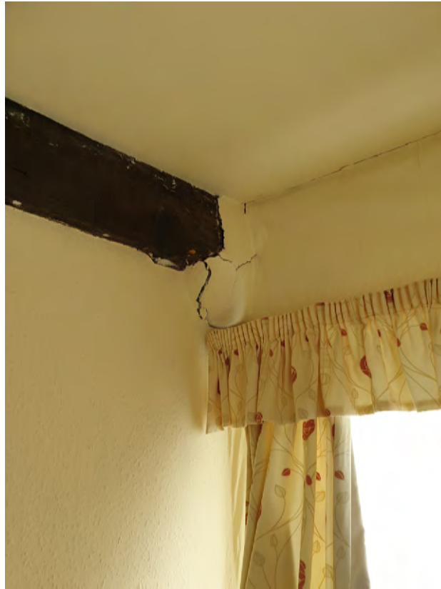
Figure 19 View of crack in first-floor room on east wall
