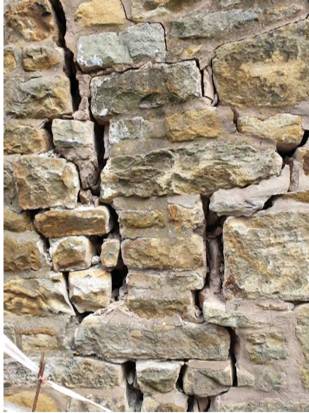
Figure 5 Detail of cracked stonework
