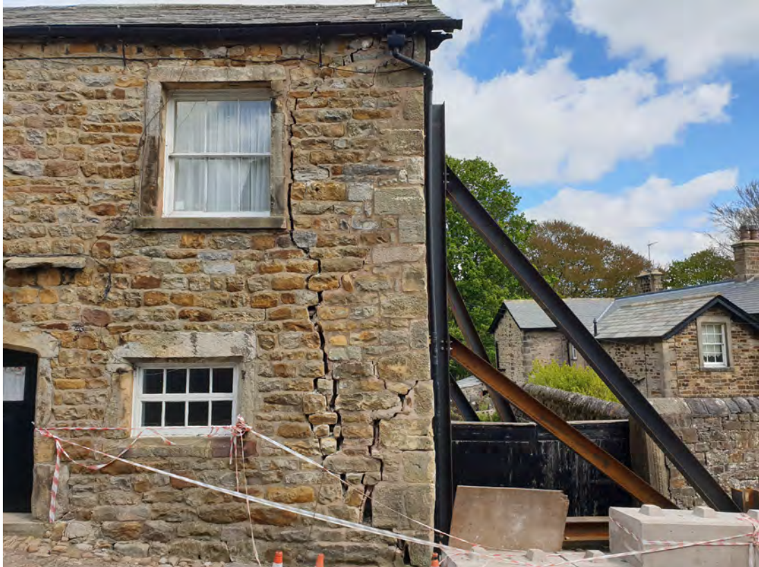
Figure 4 View of cracked stonework
