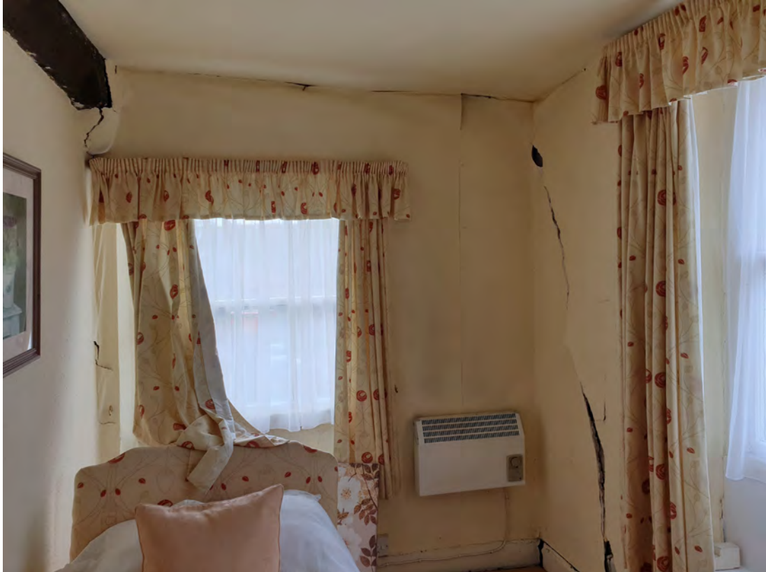
Figure 16 View of first-floor south-eastern room. Note extent of cracking to the wall and floor
