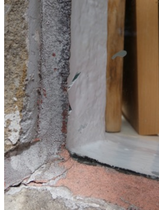
IMAGE 05 – CRACKED FLOAT GLASS TO GROUND FLOOR WINDOW
