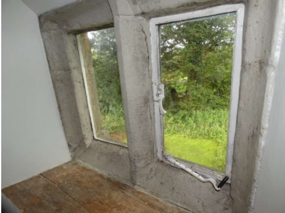
IMAGE 08 – FIRST FLOOR OPENING LIGHT WINDOW
