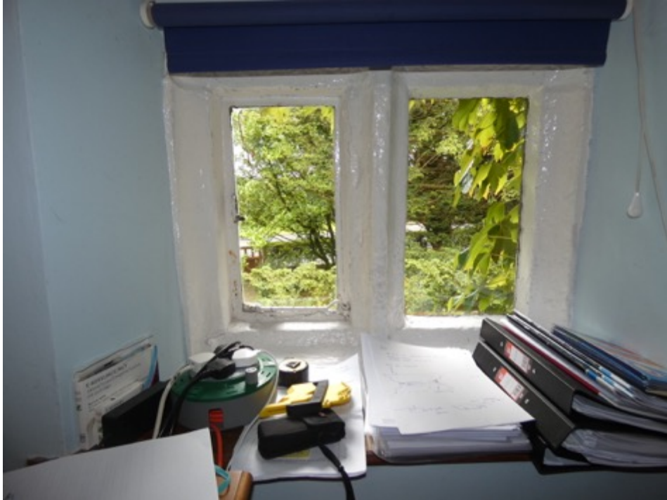
IMAGE 010 – THICK LAYERS OF PAINT TO STONE REVEALS
