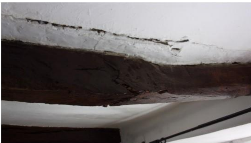
Photo 3 - View of Crack in Right Hand Beam
