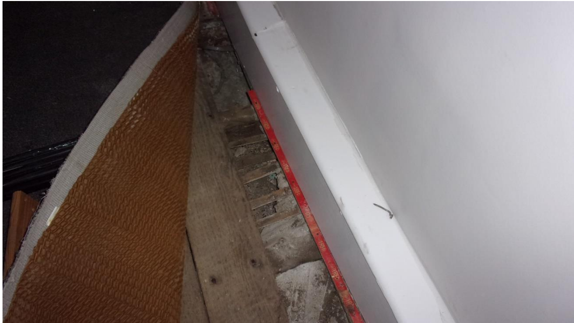
PHOTO 7 – Floor Boards and Joists Exposed in Bedroom 3
