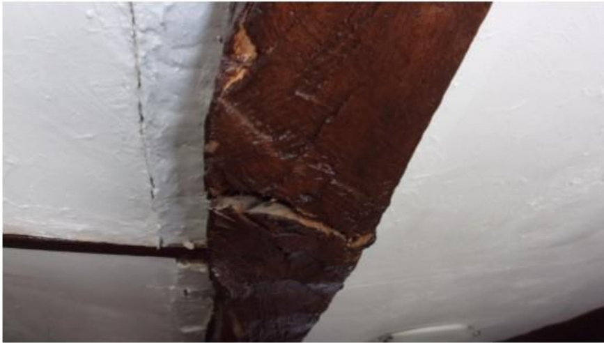
Photo 1 - View of Crack in Beam from Below
