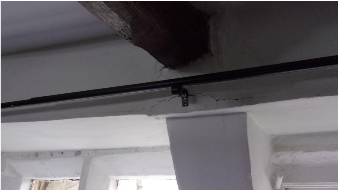
PHOTO 2- Crack at Beam Bearing
