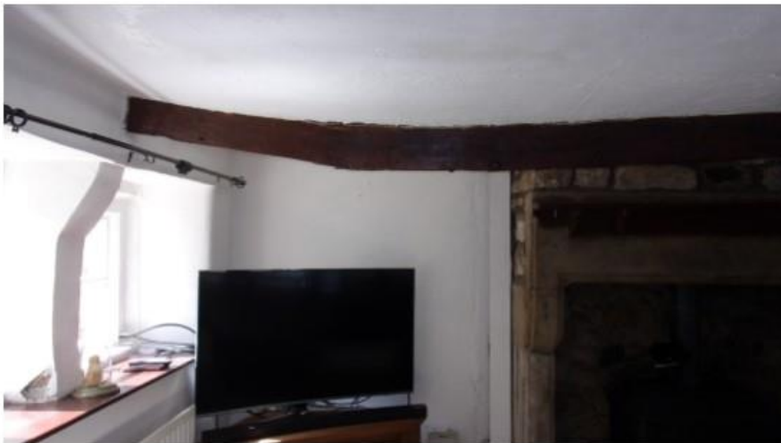
Photo 2 - View of Deflected Beam
