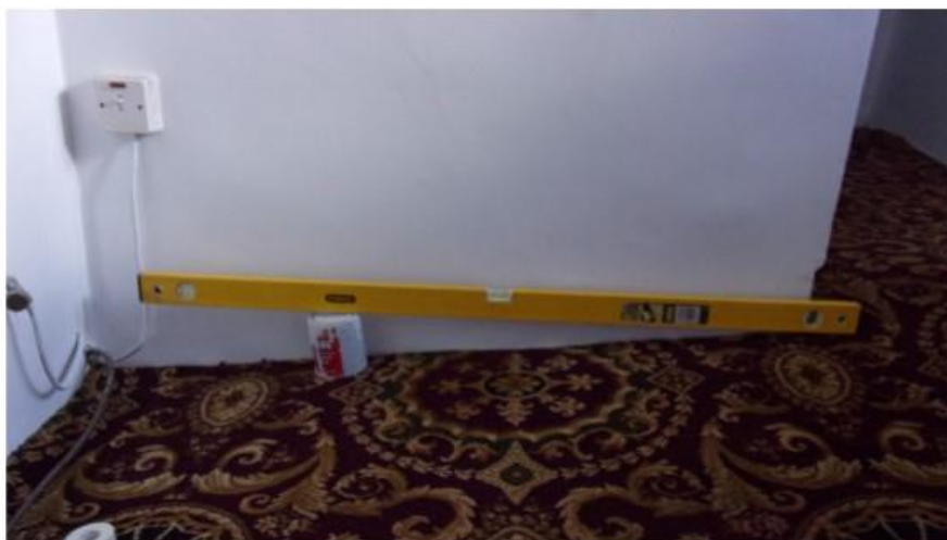
Photo 5 - Fall in First Floor at Front of Property
