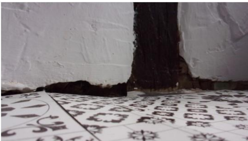
Photo 3 - View of Gap at Base of Bathroom Wall
