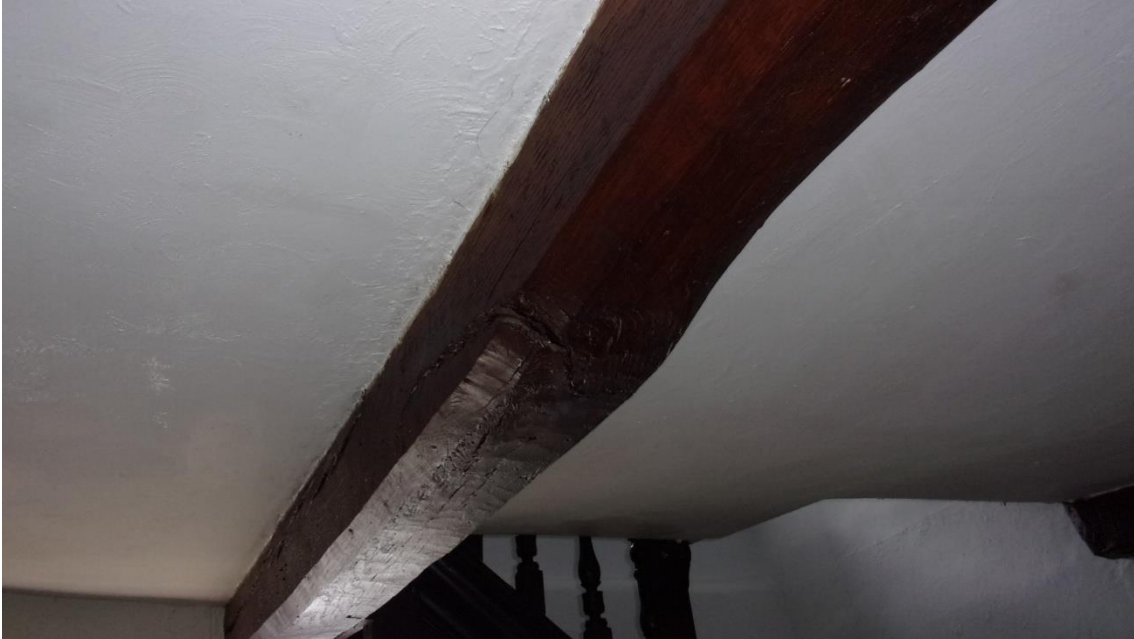
PHOTO 3 – Crack to Beam Adjacent to Staircase in Sitting Room
