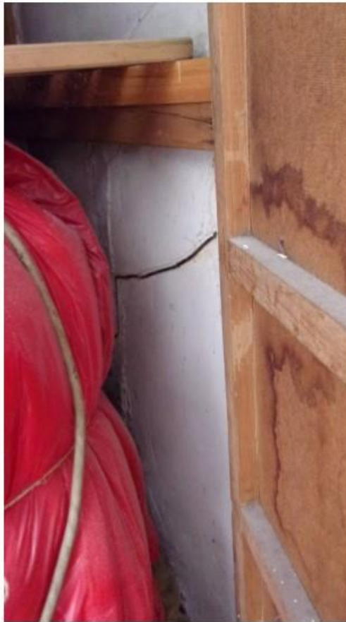
Photo 4 - View of Cracks in Partition Wall in Cupboard in Bedroom
