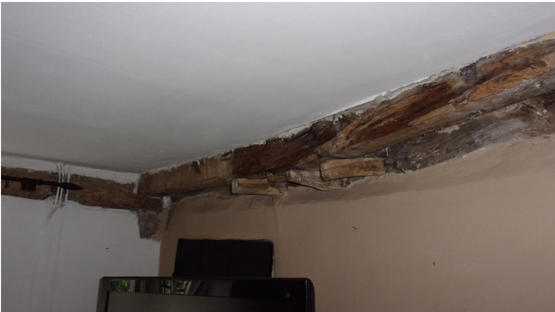
PHOTO 4 –Beam in Dining Room
