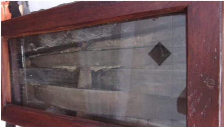
Photo 2 - Feature Panel in Bathroom Wall
