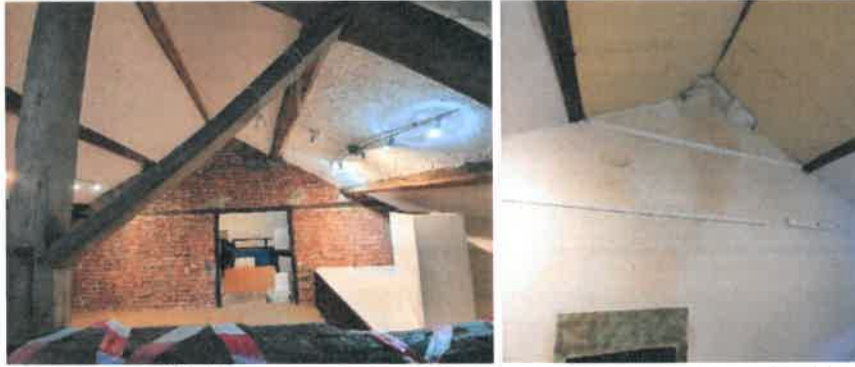
Plate 25 and 26: Red brick partition wall and gaps between ceiling and gable wall.
