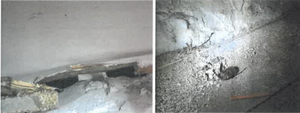
Plate 15 and 16: Large gap between wall and ceiling, deceased bat beneath the gap.
