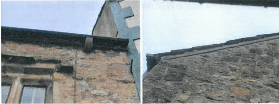
Plate 7 and 8: Gaps behind fascia board and along the roof verge.
