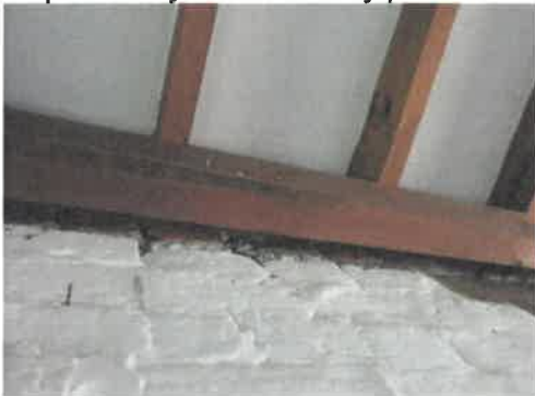
Plate 23: gaps between joists and wall.
