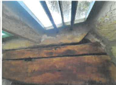
Plate 24: cracks and gaps in stone and lintel.
