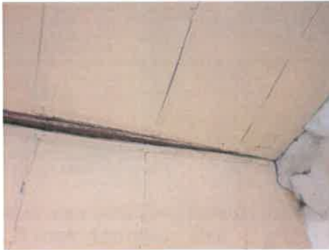
Plate 27: Gap between ridge board and insulation boarding.
