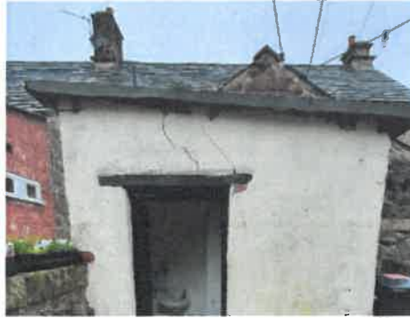
Plate 10: Extension 2 with lifting roof felt.
