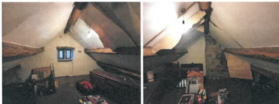
Plate 13 and 14: Gable end with window and partition wall with stone chimney breast.
