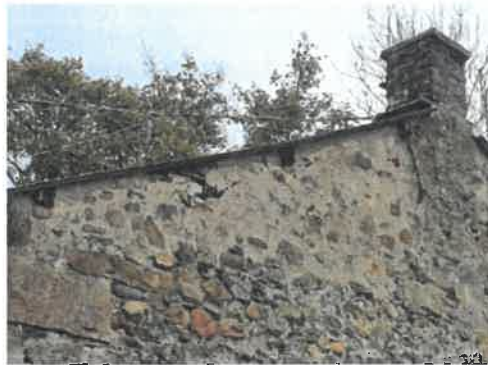
Plate 11: Gaps in stonework and mortar.
