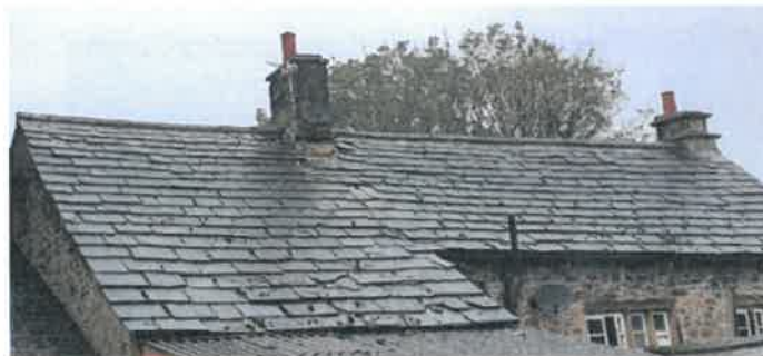
Plate 9: Broken roof tiles and lifted lead flashing to the rear of the property.
