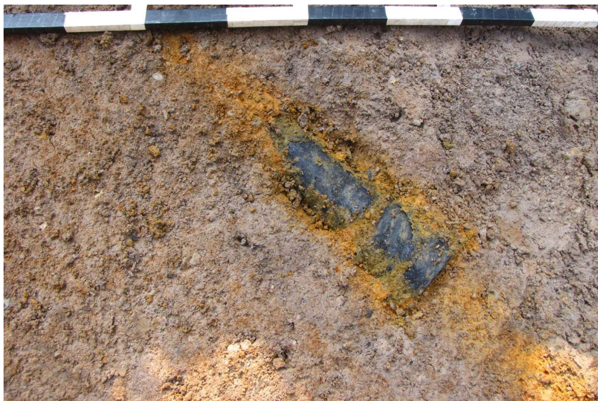
Plate 8. Modern cast iron or steel water pipe cut into base of excavation trench
