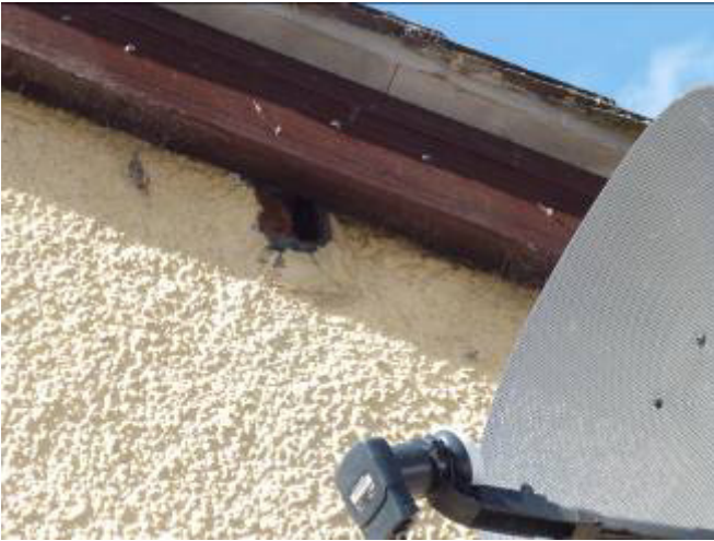
Small hole on east elevation rendered wall requires precautionary inspection with torch / endoscope.
