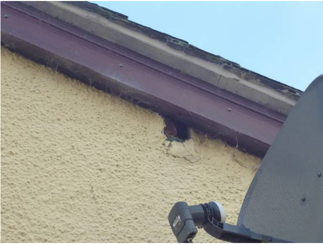
Small hole on east elevation rendered wall requires precautionary inspection with torch / endoscope.
