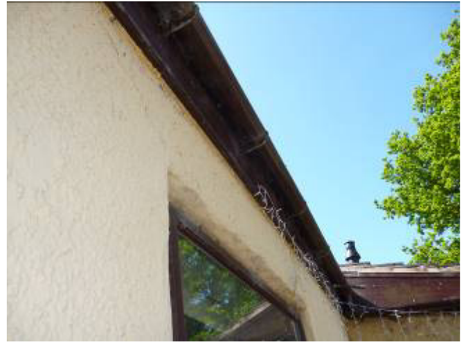
Fascia boards tight fitting / sealed against render.
