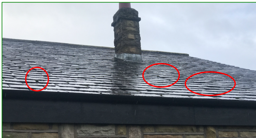
Showing a small number of crevices under slates on the northeast elevation of the garage
