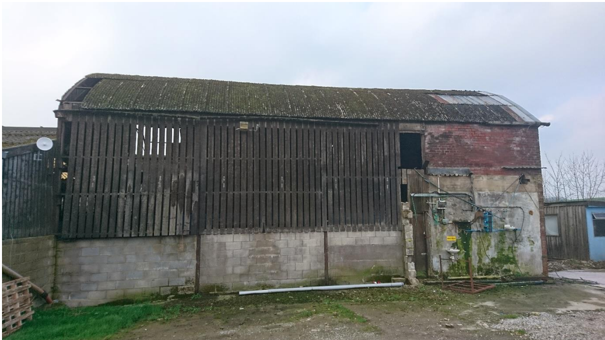
Figure 7: View of the northern elevation showing the partial masonry and steel/timber cladding construction
