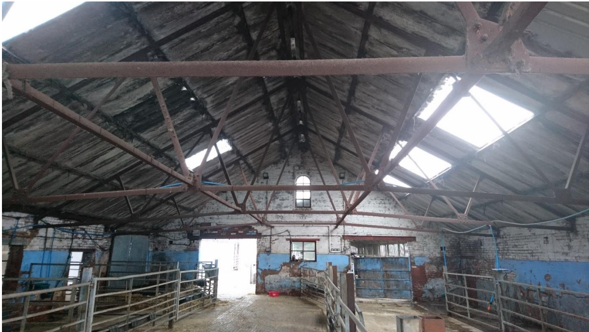
Figure 5: Internal view of the pitched roof structure, noting longitudinal restraints to truss chords
