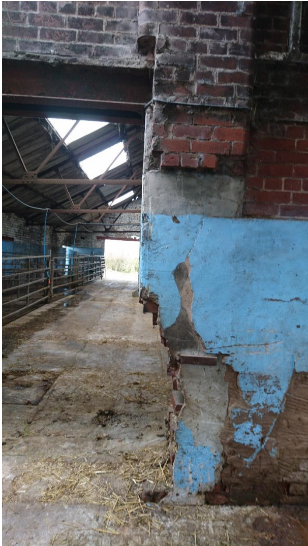
Figure 17: Damaged masonry at opening O6
