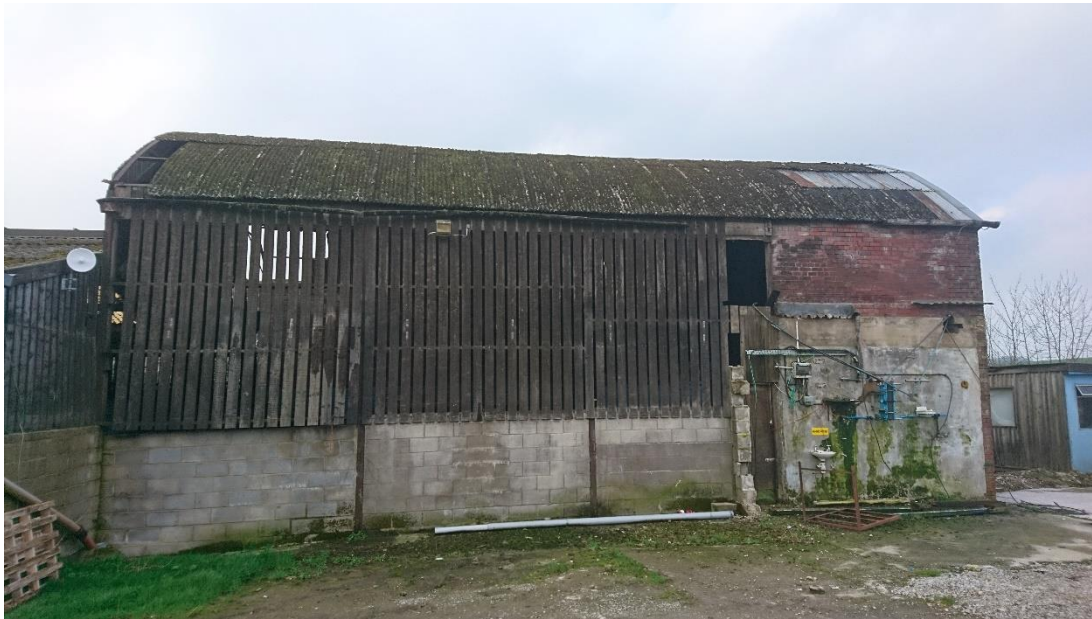
Figure 2: View of the northern elevation showing the partial masonry and steel/timber cladding construction
