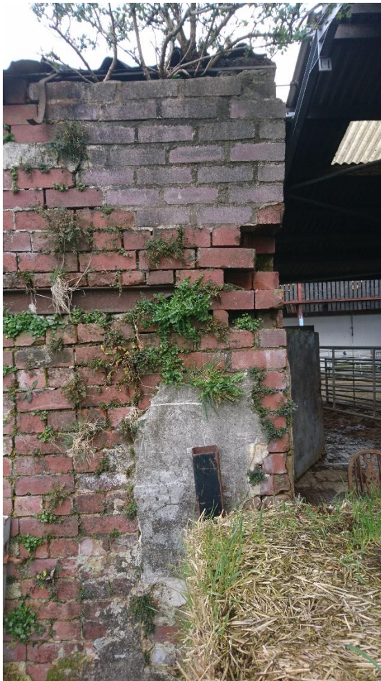
Figure 13: south eastern corner of pitched barn in disrepair
